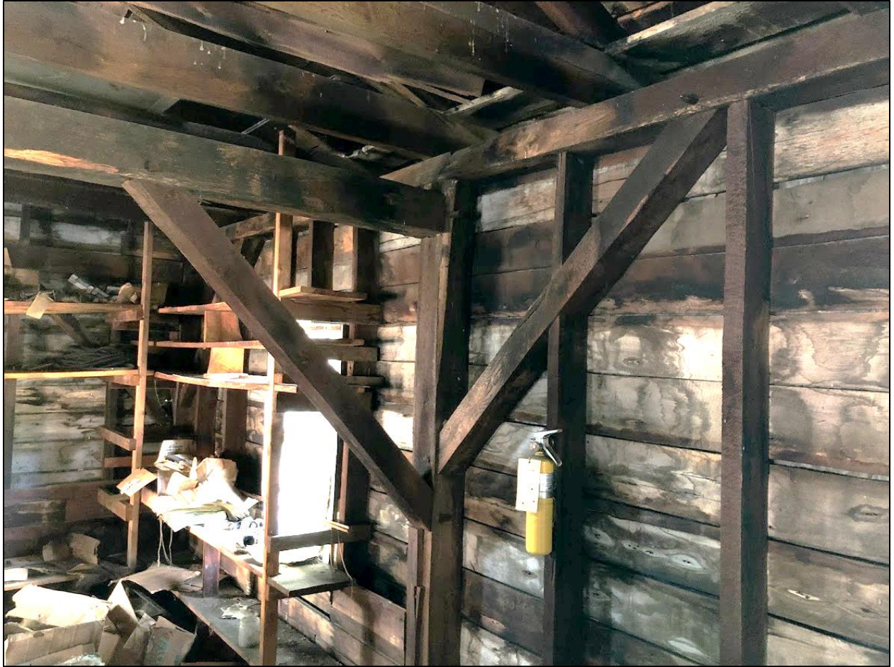
11. Smith Hoyle's Mill, Second floor interior view of original timber-framing in building's southeast corner that was expanded eastward by one bay.
