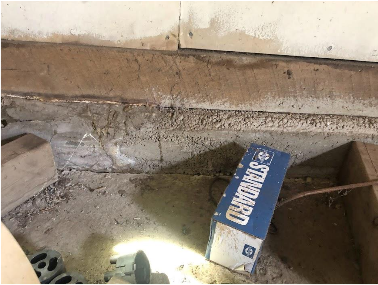
39. White Barn, West room, south wall interior concrete foundation detail. Photo number 7285.
