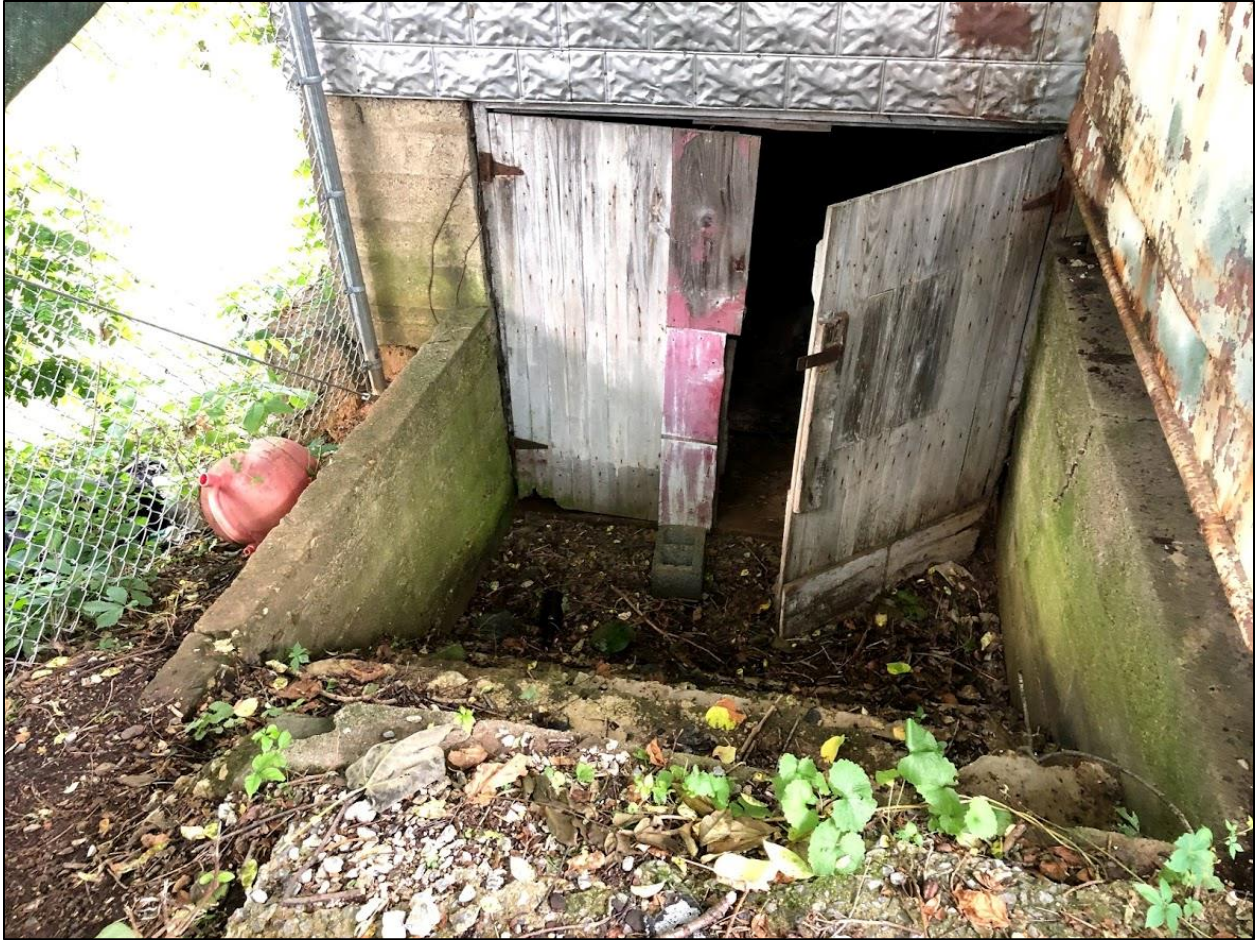
14. Smith Hoyle's Mill, View down to basement doors on east elevation at building's southeast corner.
