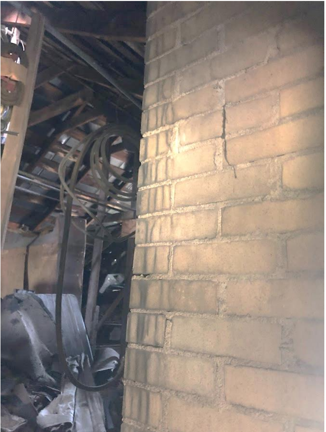
53. White Barn, Second floor loft, view in from north elevation window. Photo number 7242.
