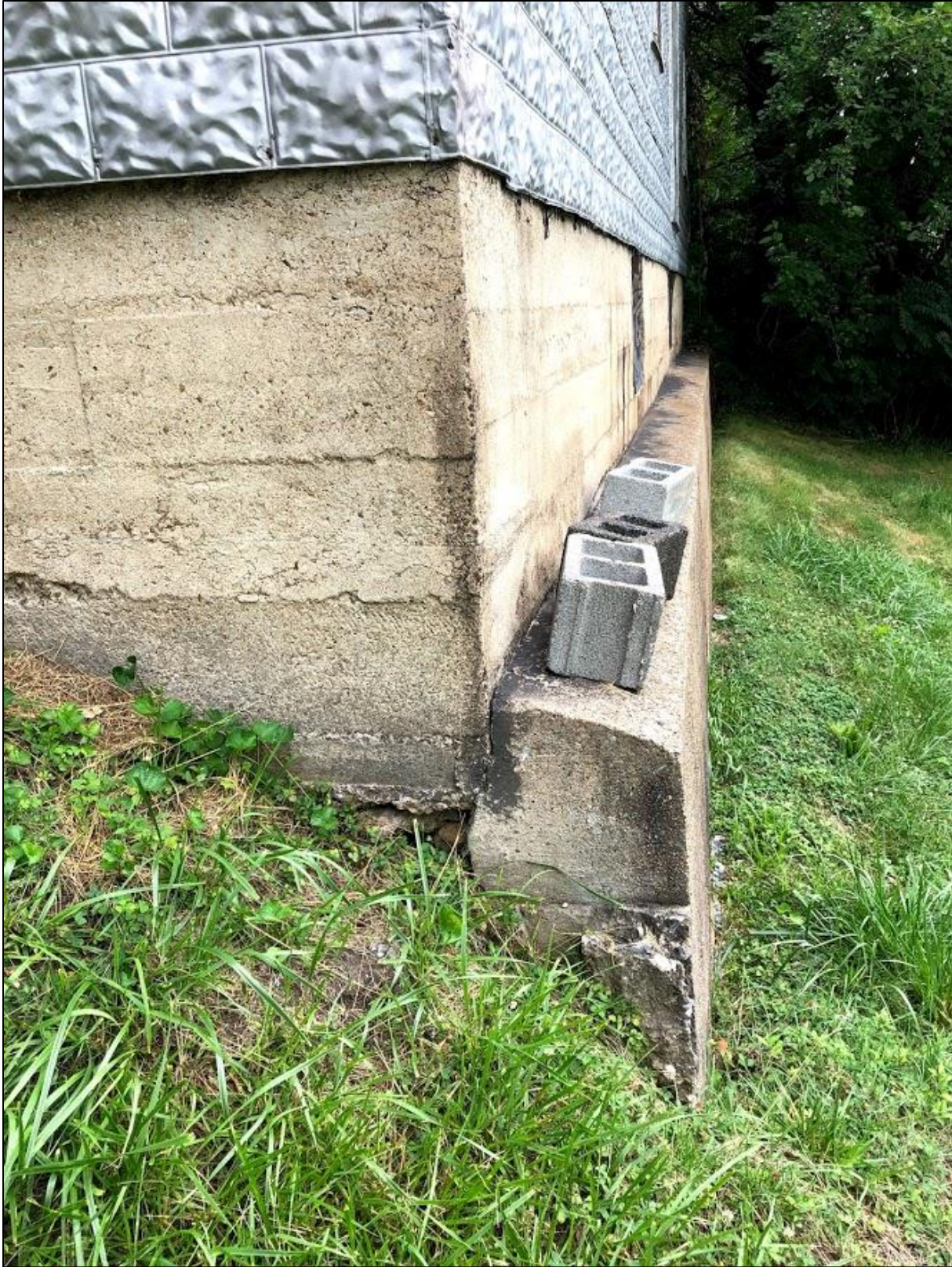
5. Smith Hoyle's Mill, Southwest corner of cast-in-place concrete foundation on earlier masonry foundation with concrete buttress along entire length of south elevation.
