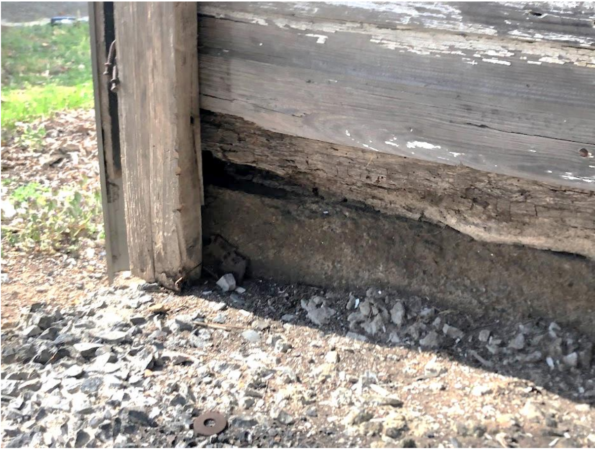
21. White Barn, View south to wood sill plate at east end of north elevation. Photo number 7199.
