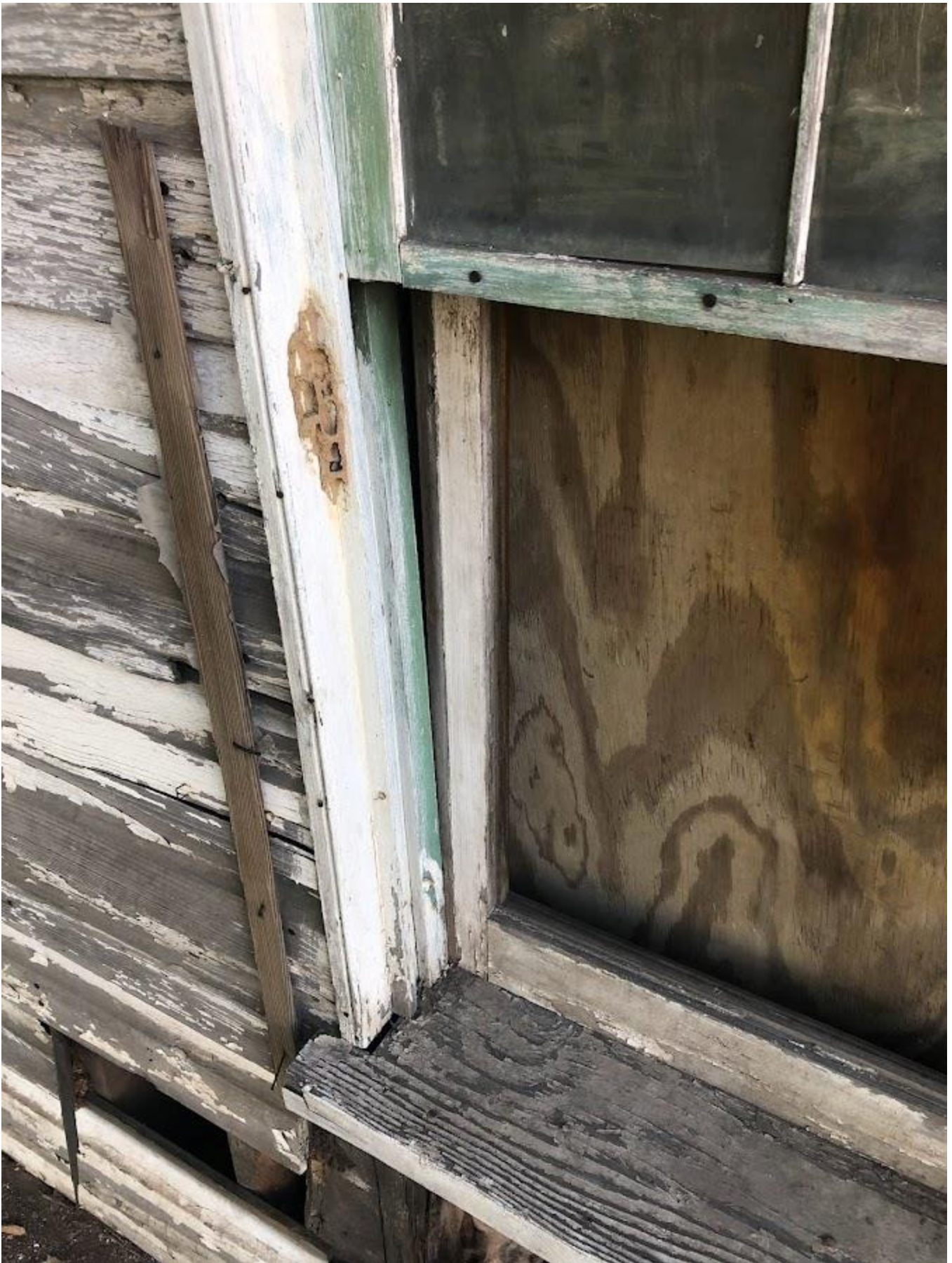
26. White Barn, First floor window meeting rail, jamb, and sill detail. Photo number 7175.
