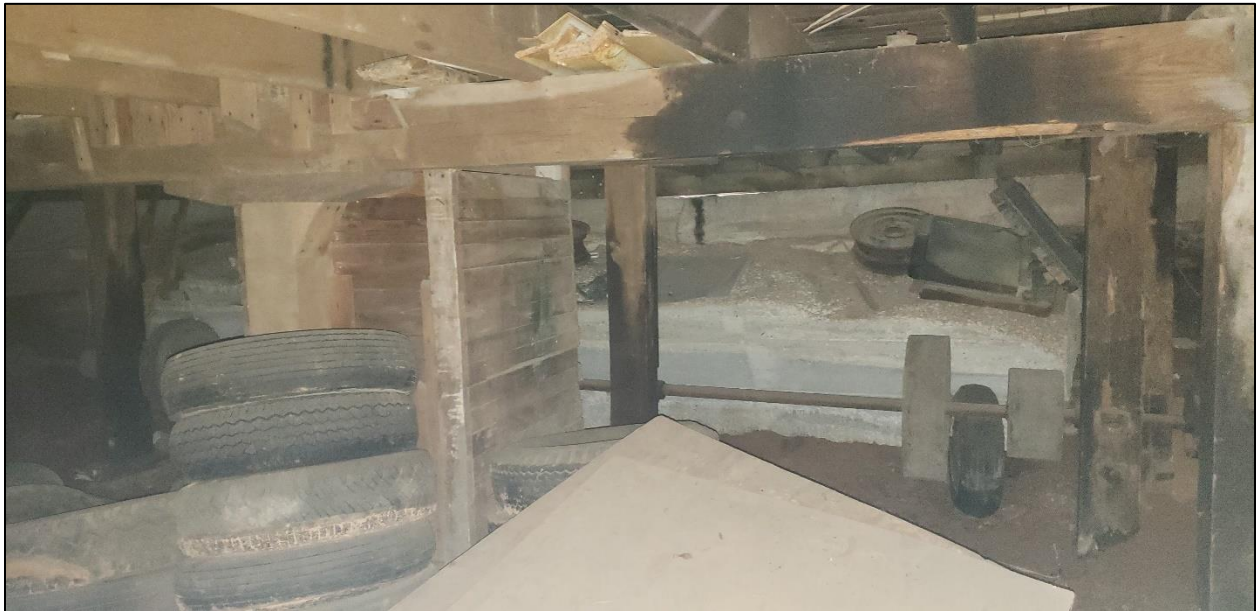
18. Smith Hoyle's Mill, Basement interior view north to shaft wheels (to run fan-belts to power the milling equipment) in front of concrete buttress against north foundation.
