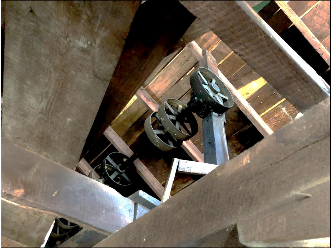
13. Smith Hoyle's Mill, Second floor interior view up to attic showing original shaft wheels to run fan-belts to power the milling equipment.
