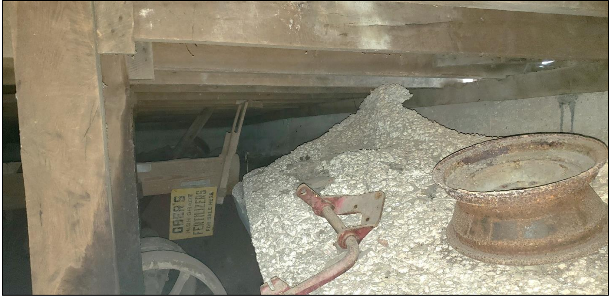
19. Smith Hoyle's Mill, Basement interior view west along north foundation showing the concrete buttress overturning due to soil settlement below (shaft wheels at lower left remain in place to run fan-belts to power the milling equipment).
