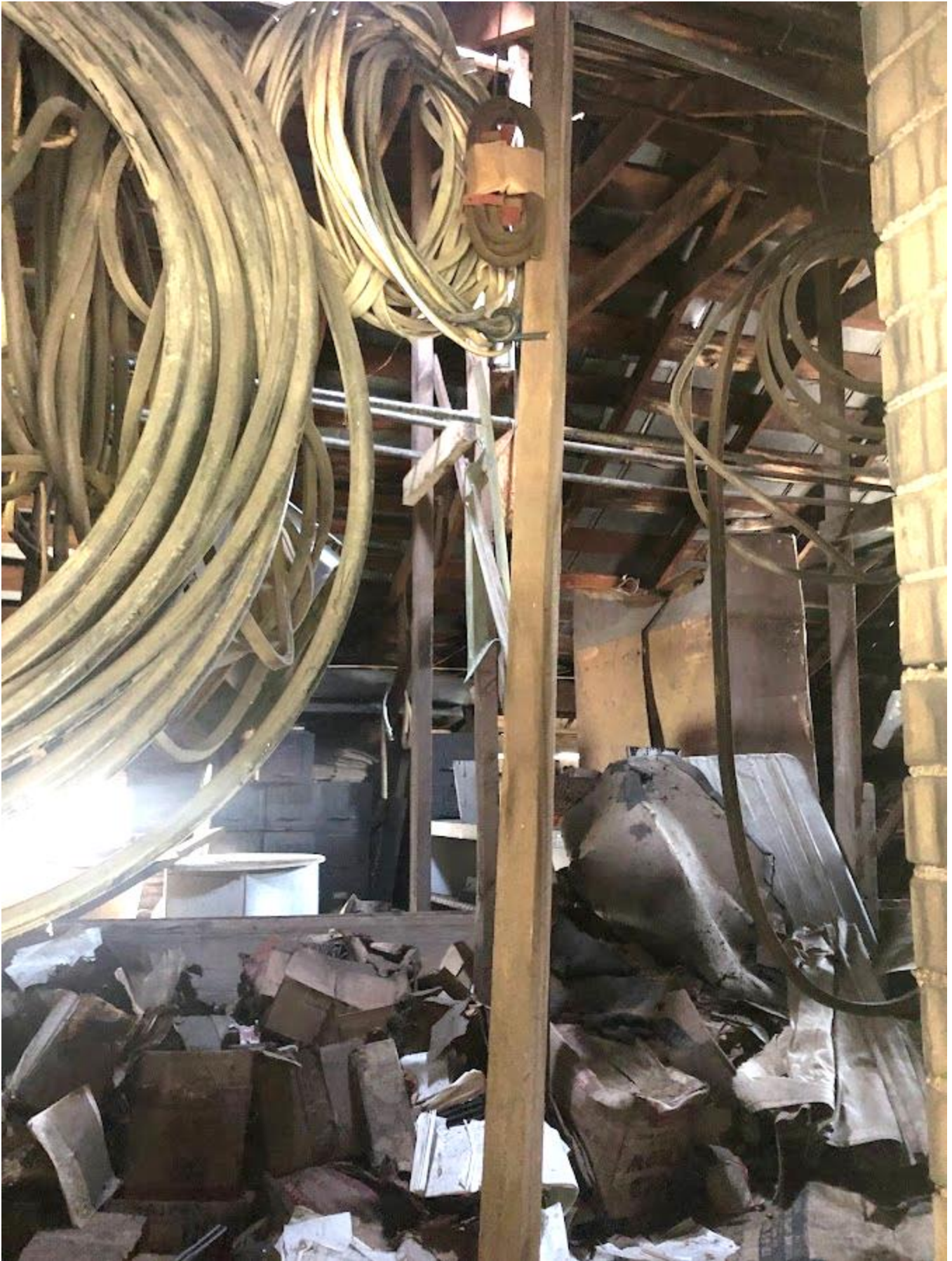
51. White Barn, Second floor loft, view in from north elevation window. Photo number 7237.
