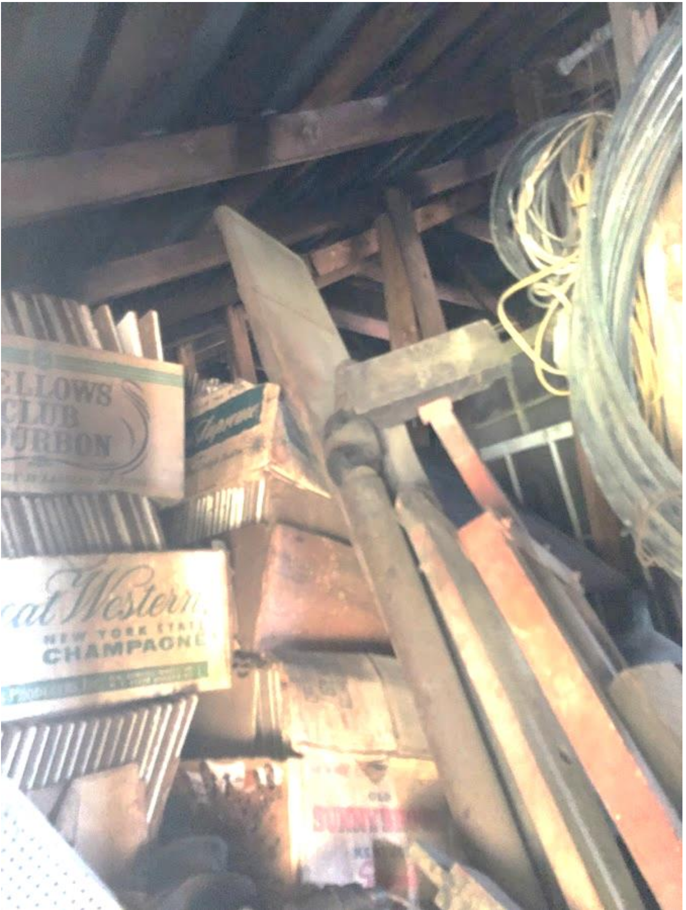
48. White Barn, Second floor loft, view in from north elevation window. Photo number 7240.
