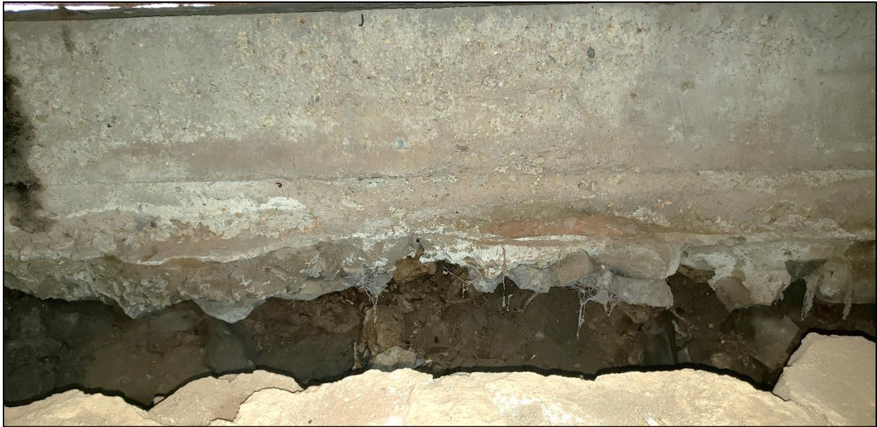
20. Smith Hoyle's Mill, Basement interior view to north foundation revealing the lower masonry wall has washed out, and the concrete buttress placed alongside the north foundation has shifted away by a few feet.
