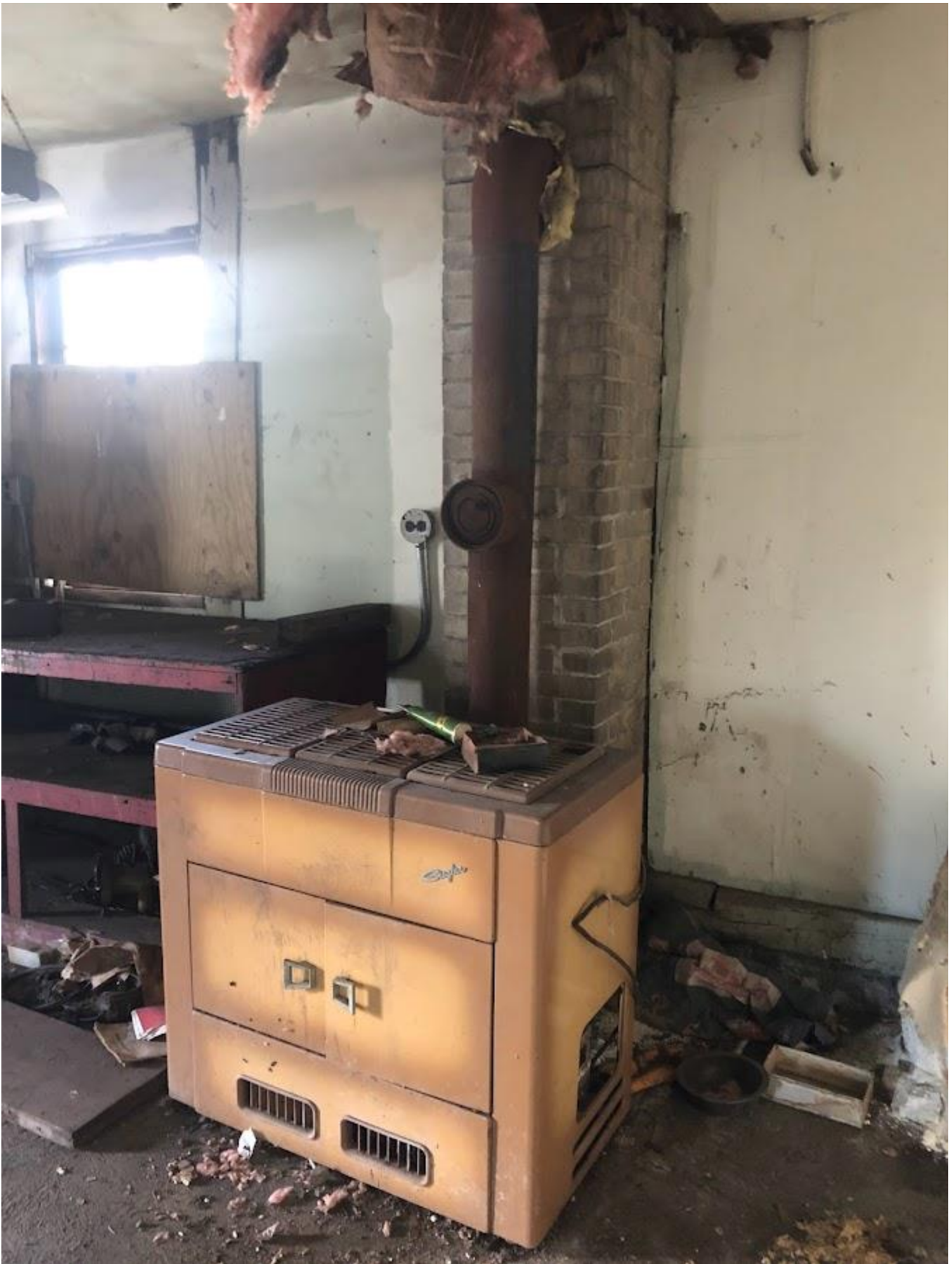
36. White Barn, West room, heating unit detail. Photo number 7262.
