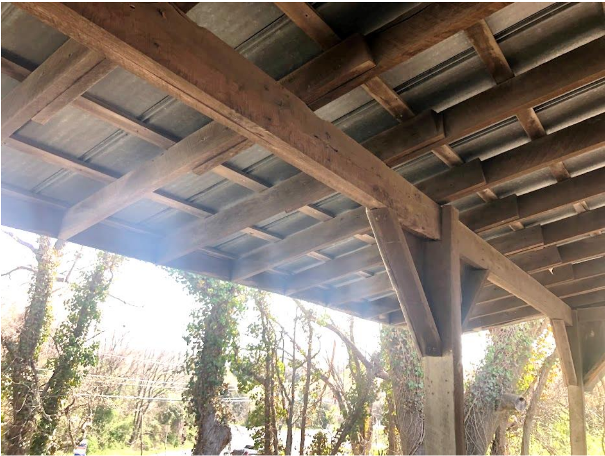
17. White Barn, View northeast to truck port overhang and two easterly support posts. Photo no. 7191.
