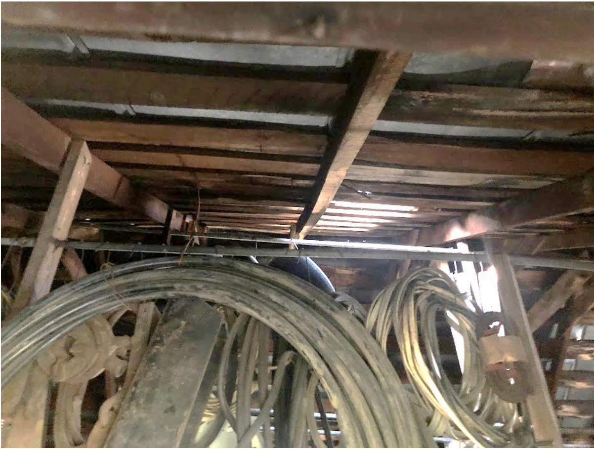
54. White Barn, Second floor loft, view in from north elevation window. Photo number 7247.
