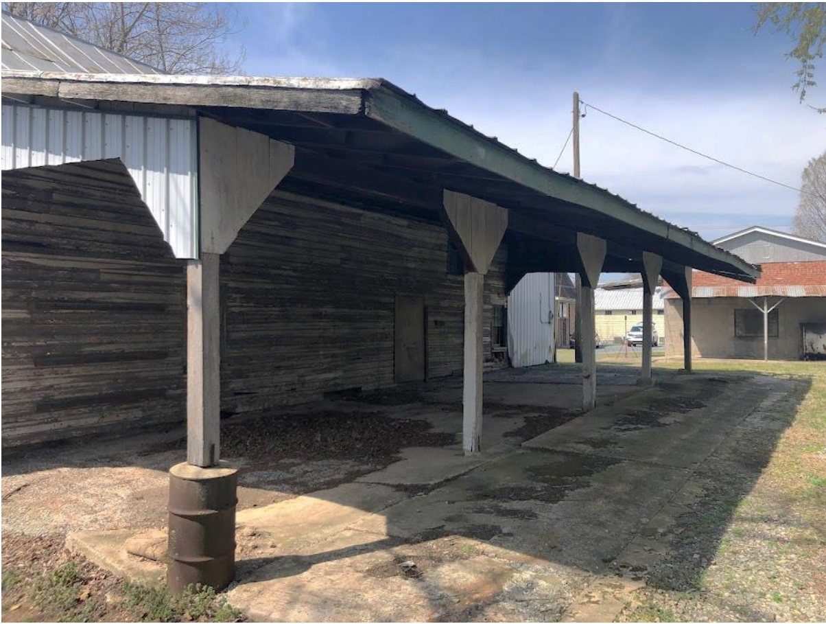
5. White Barn, View west at overhang of truck port at north elevation. Photo number 7295.
