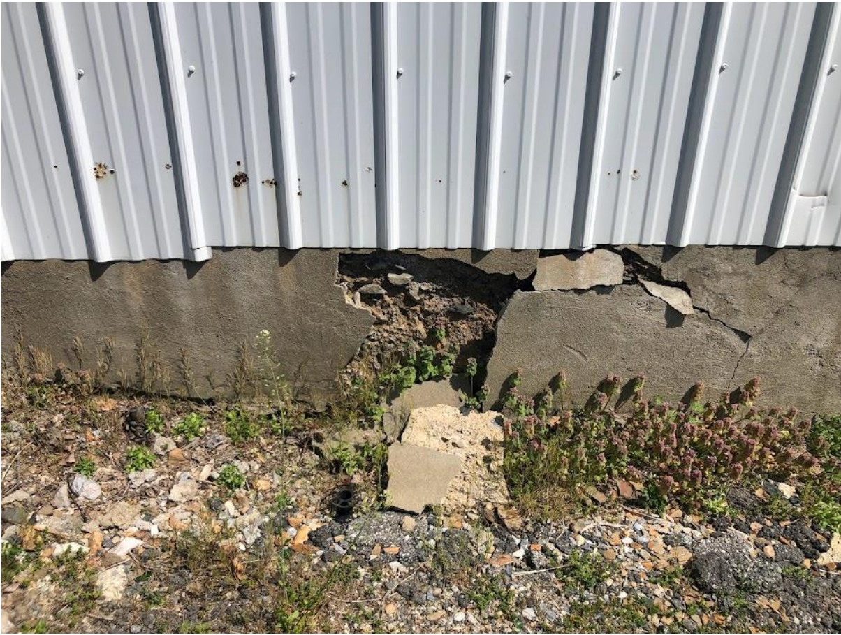
23. White Barn, View north to south foundation spalling concrete. Photo number 7299.
