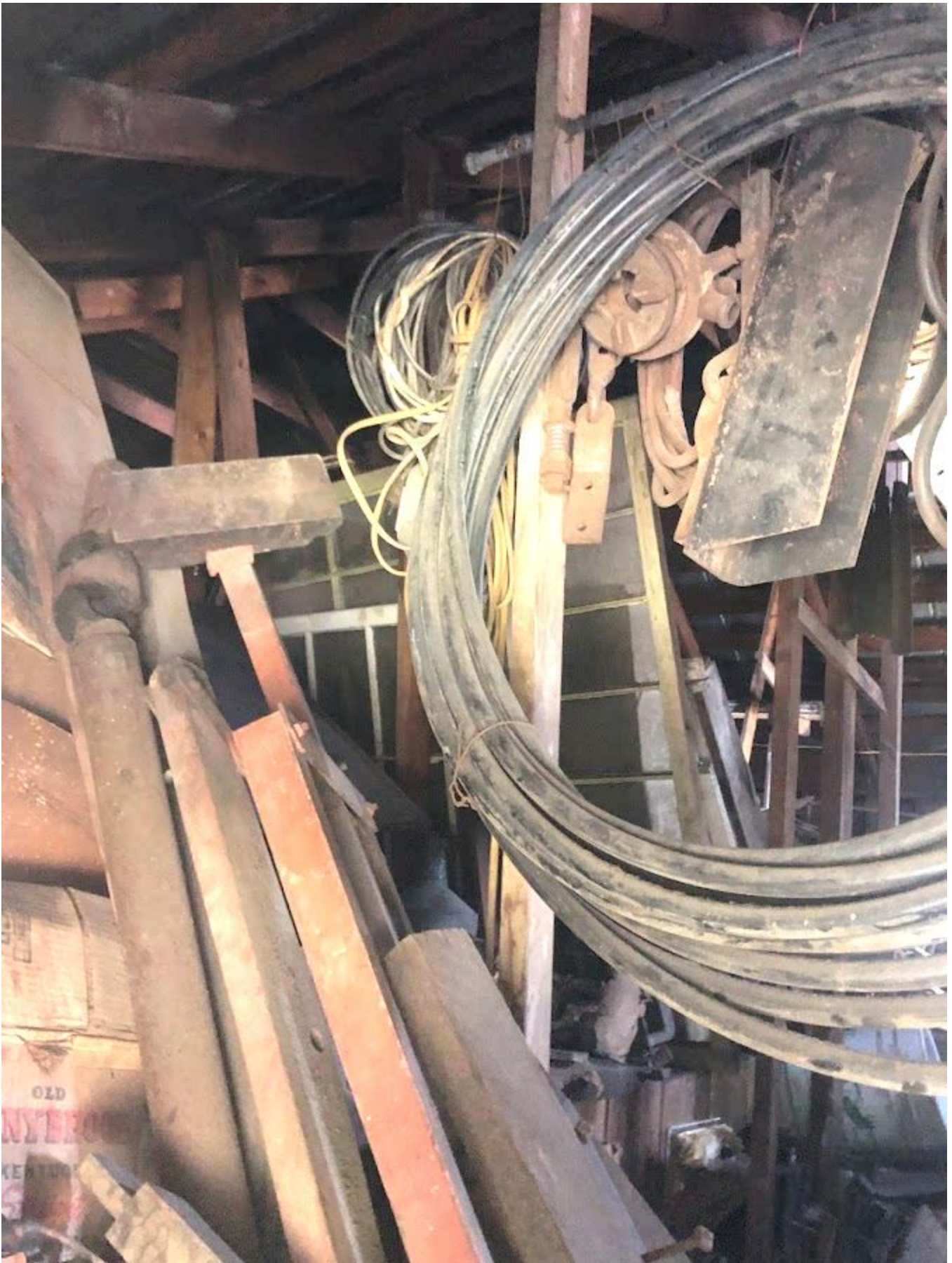
49. White Barn, Second floor loft, view in from north elevation window. Photo number 7239.
