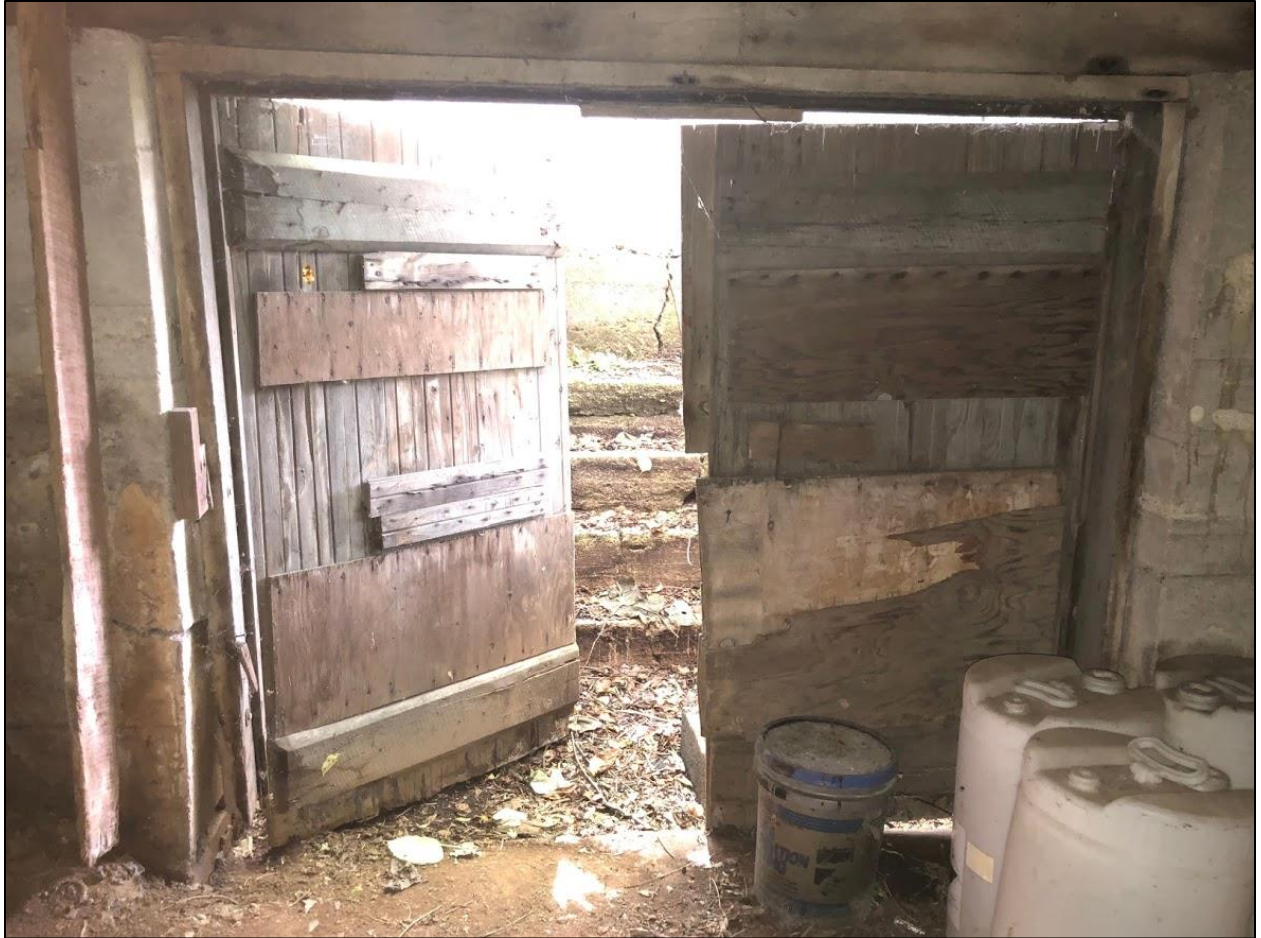
15. Smith Hoyle's Mill, Basement interior view east to interior side of basement doors.
