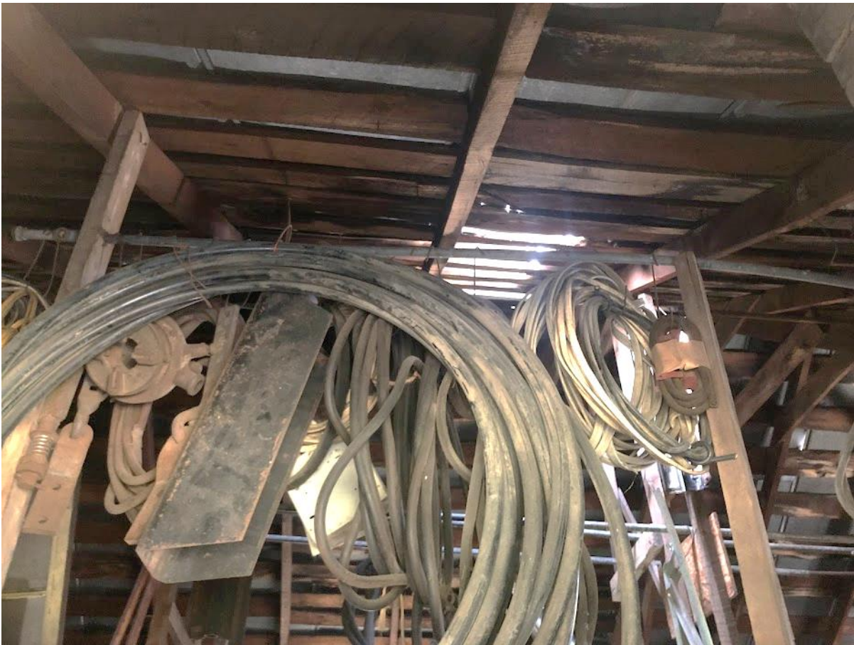
55. White Barn, Second floor loft, view in from north elevation window. Photo number 7241.
