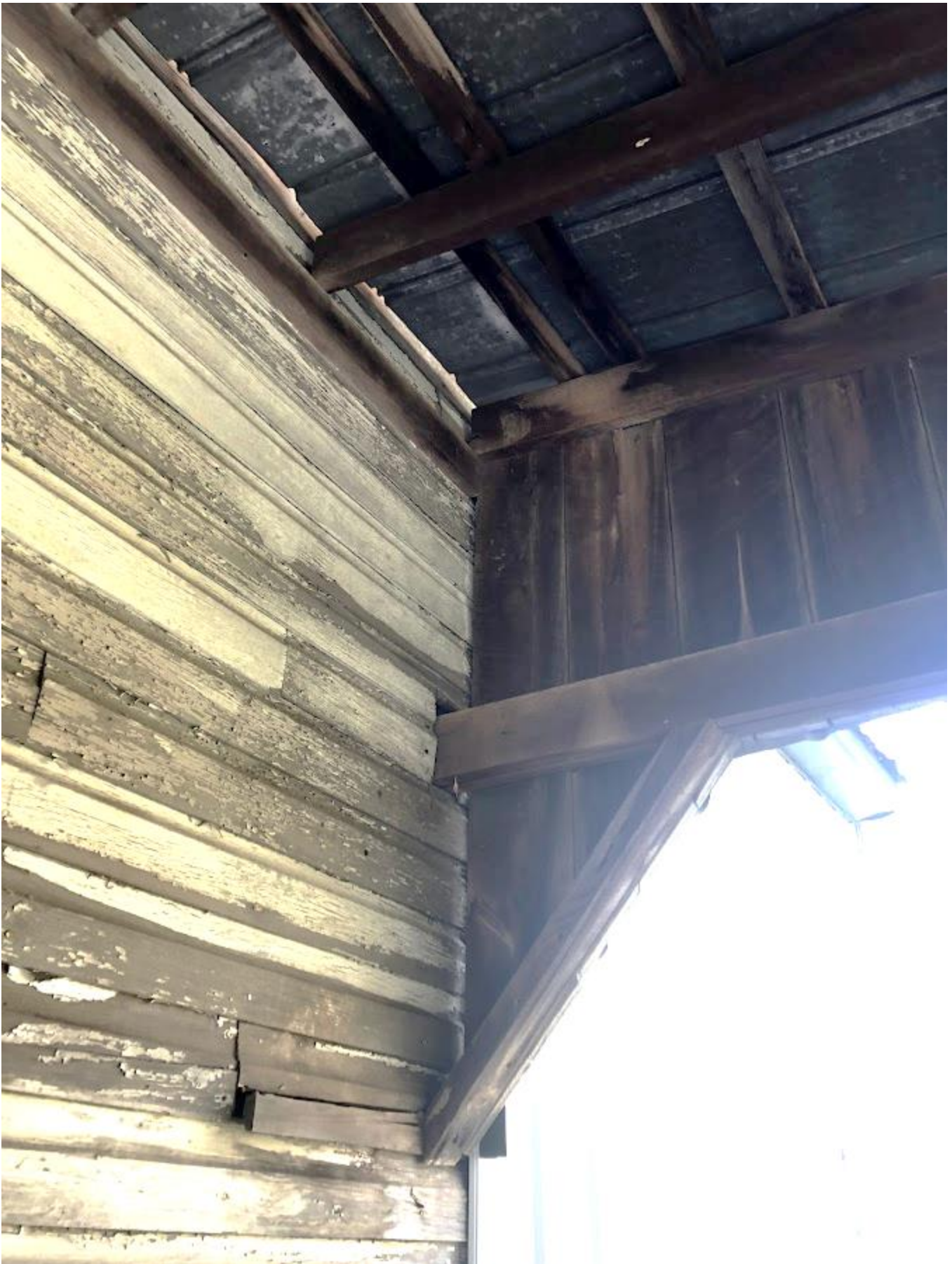
13. White Barn, View west to truck port framing into north elevation. Photo number 7187.
