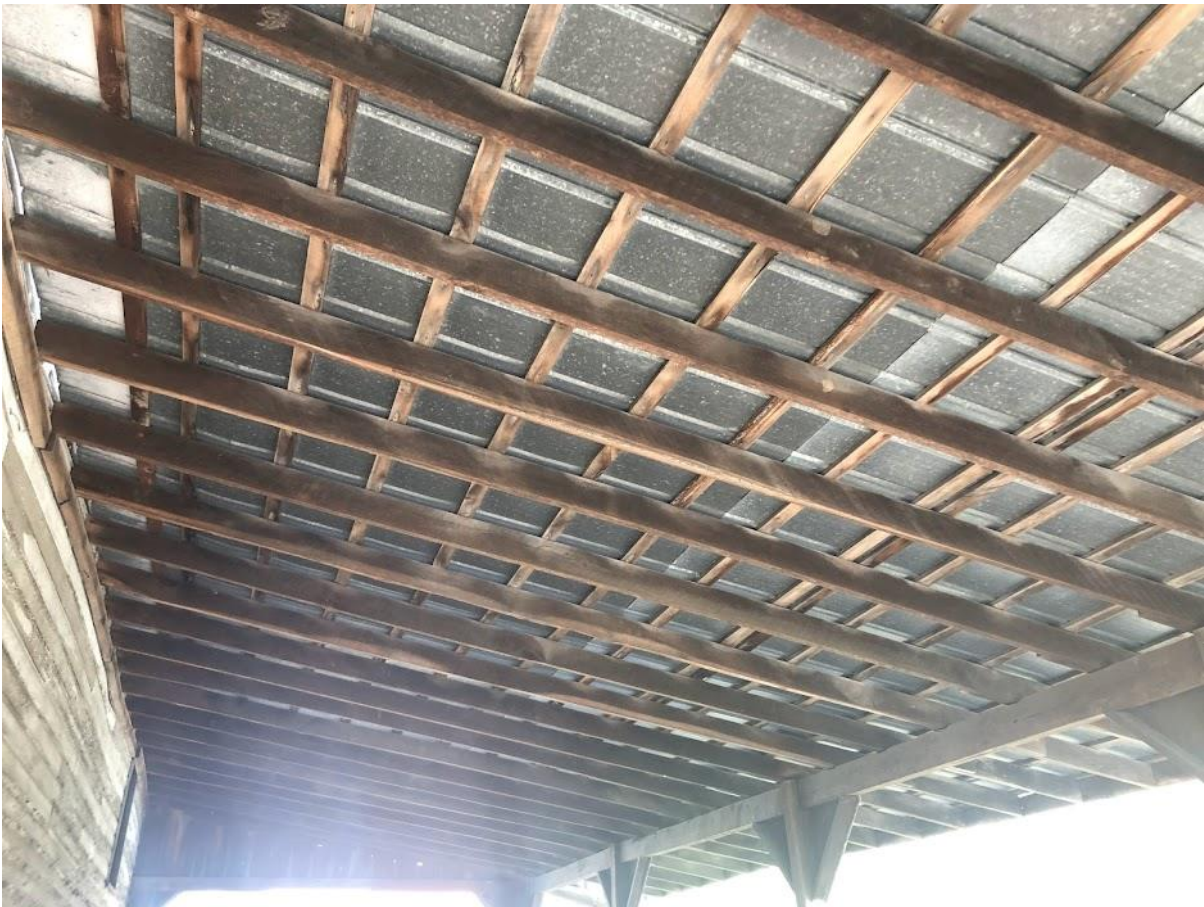
12. White Barn, View west up to truck port roof framing. Photo number 7183.
