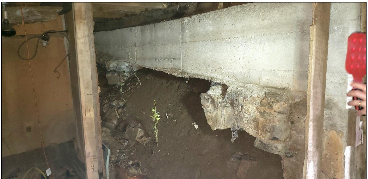
16. Smith Hoyle's Mill, Basement interior view to failed section of east foundation with dirt spilling inward.
