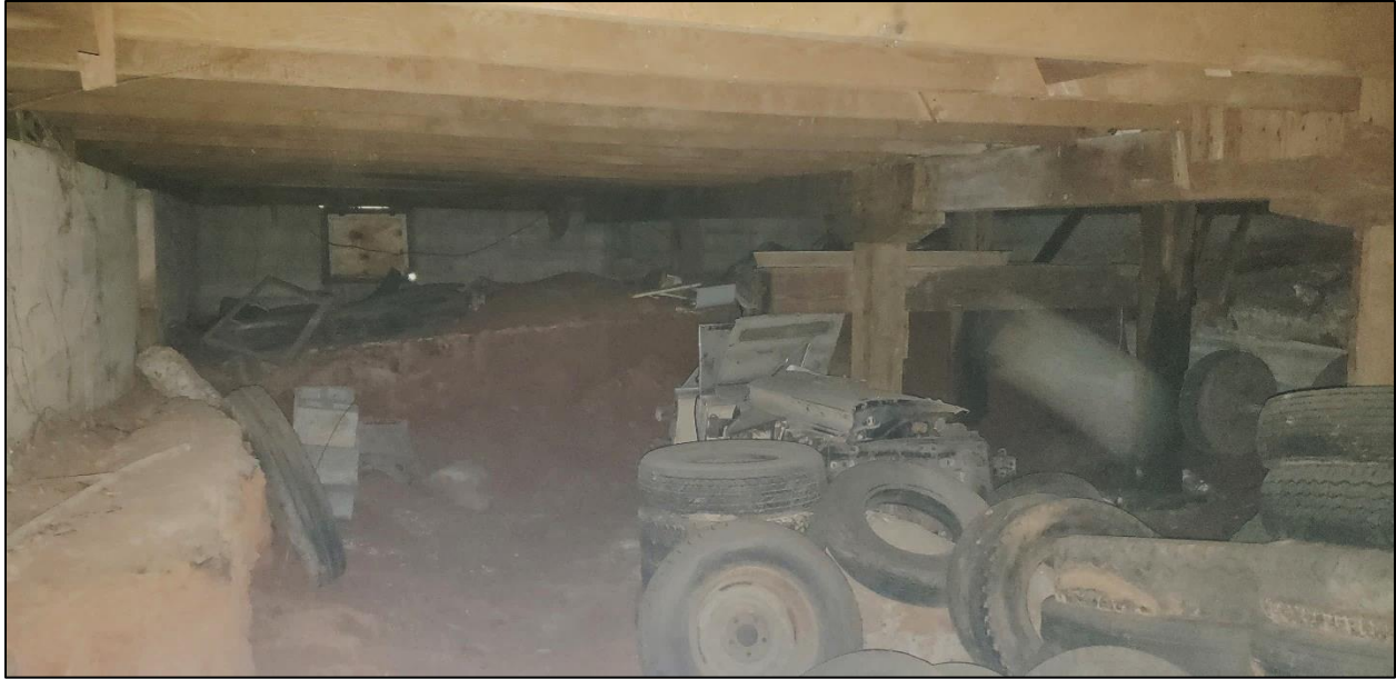
17. Smith Hoyle's Mill, Basement interior view west showing original grade and lower excavated grade.
