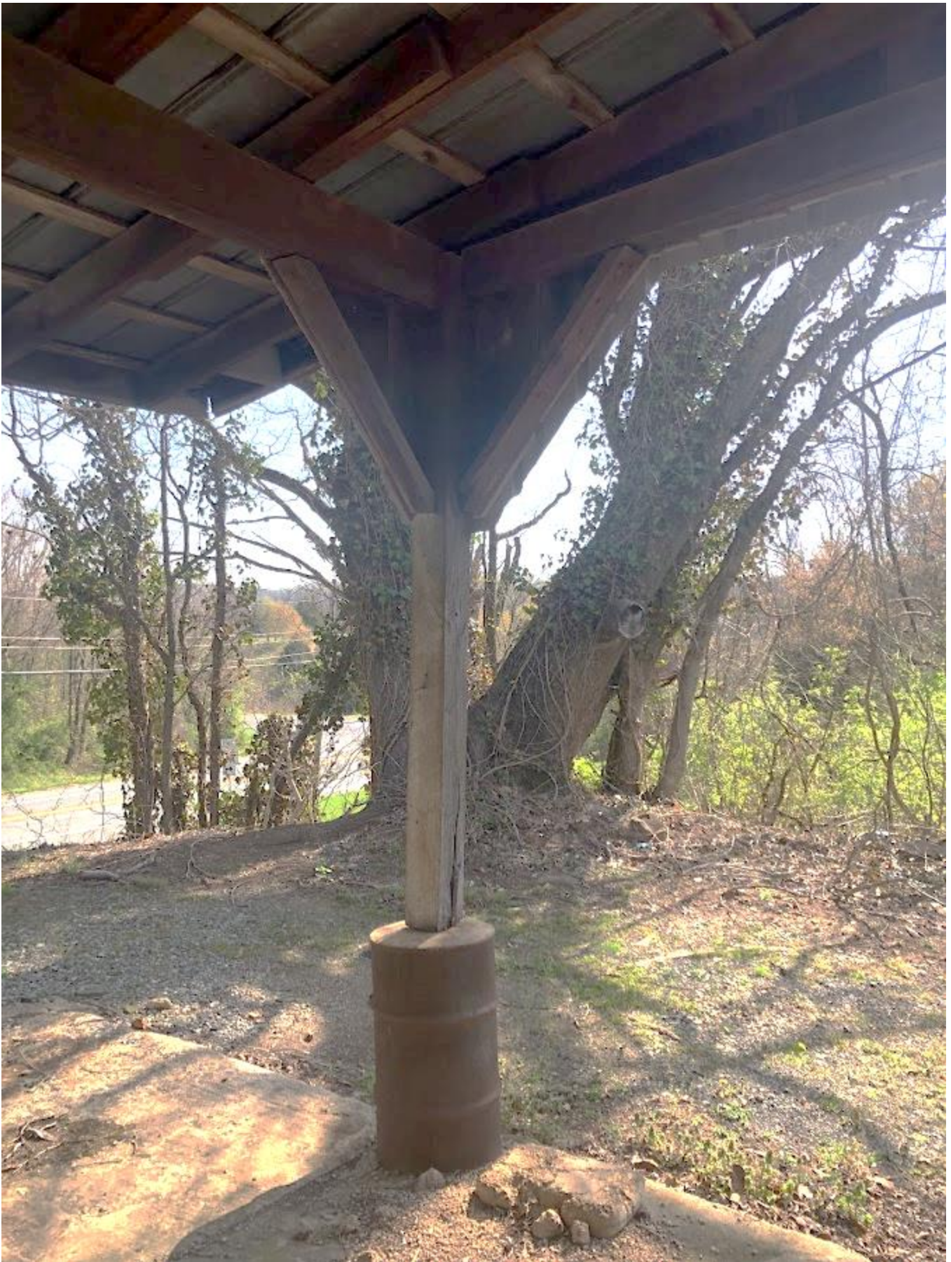
18. White Barn, View northeast at interior of easternmost support post. Photo number 7195.
