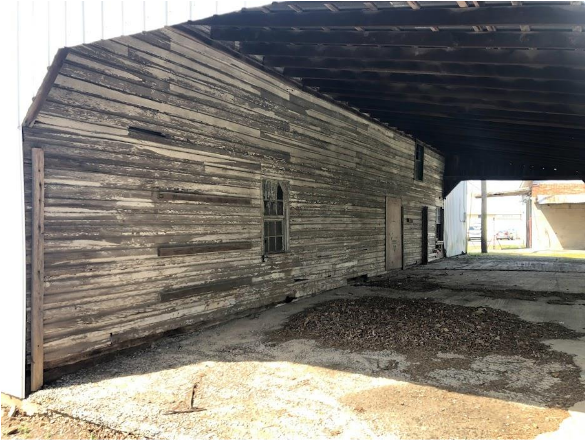
6. White Barn, View west at truck port interior north elevation. Photo number 7297.
