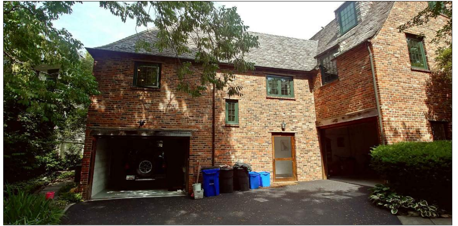
VIEW OF REAR 1-STORY WING WHERE ADDITION WILL TIE INTO EXISTING HOUSE
