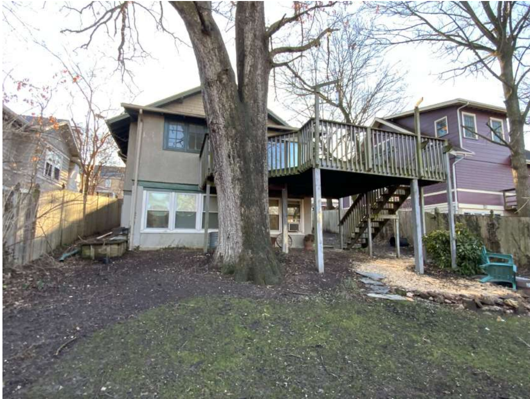
Detail: 7338 CARROLL REAR (TREE HAS BEEN REMOVED)
