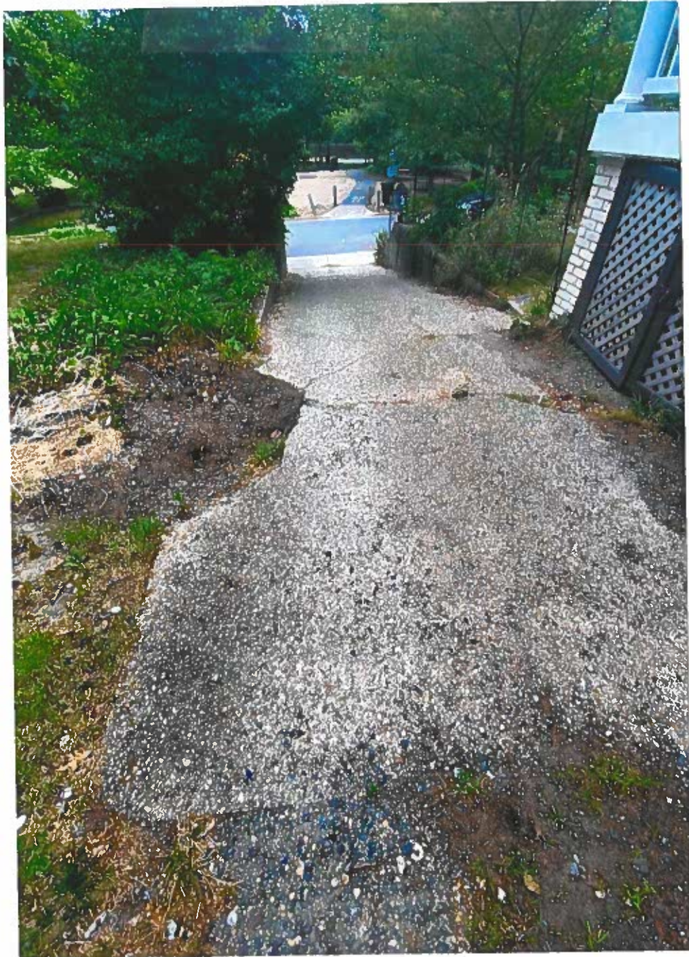
Existing damage driveway
