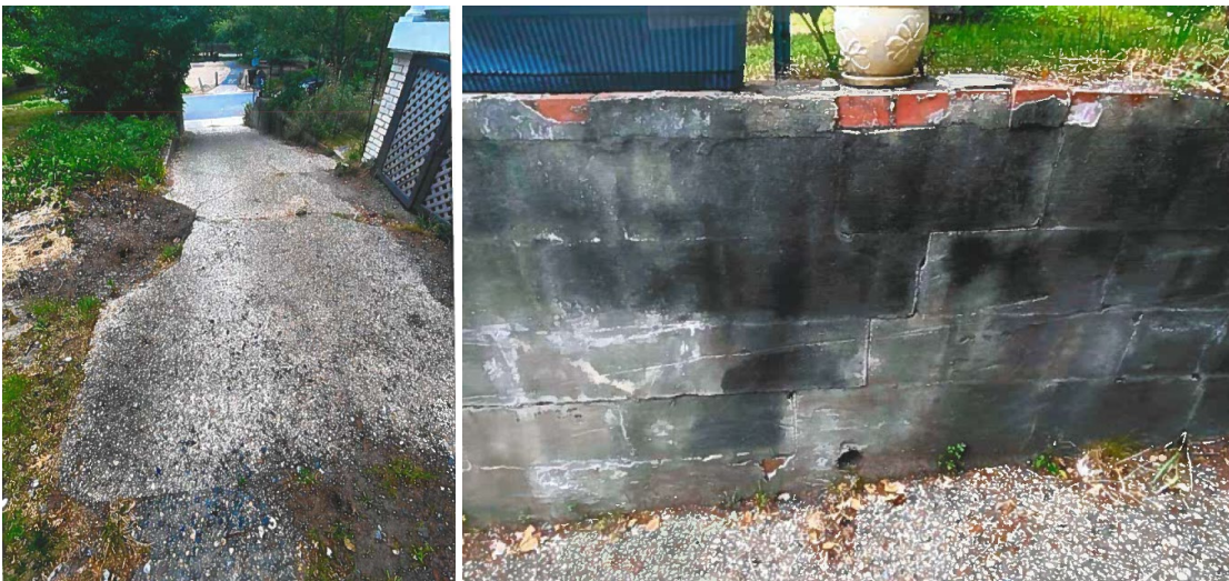
Figure 3: View of the section of driveway (left) and retaining wal (right) to be replaced, 2023. Source: Applicant.
