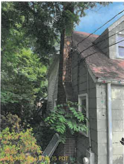
Utility Side Before Installation
