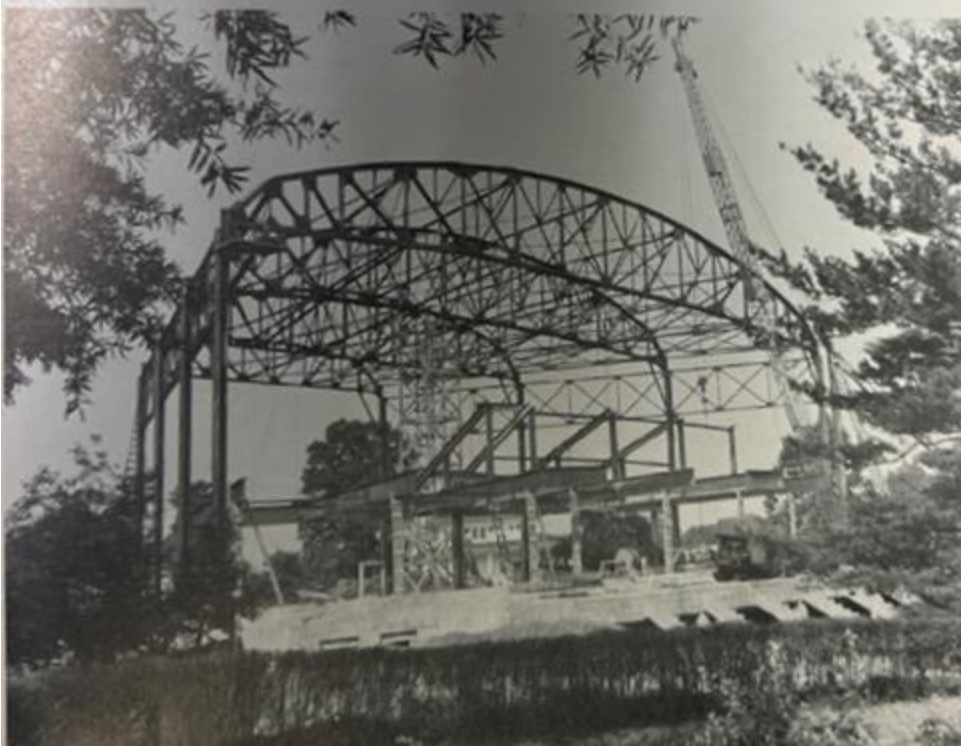
Figure 8: The Sligo Church under construction amid WWII, June 24, 1943. Source: Kitt Watts, Our Sligo , Sligo Seventh-day Adventist Church, 1974: 9.
