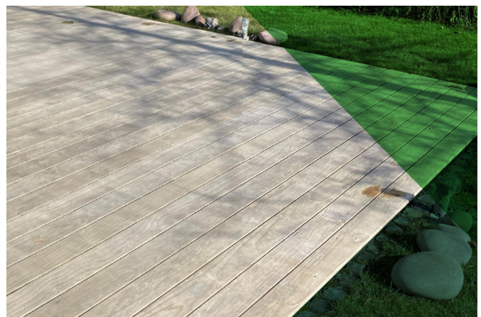
Decking in Germany after 10 years of greying and regular cleaning
