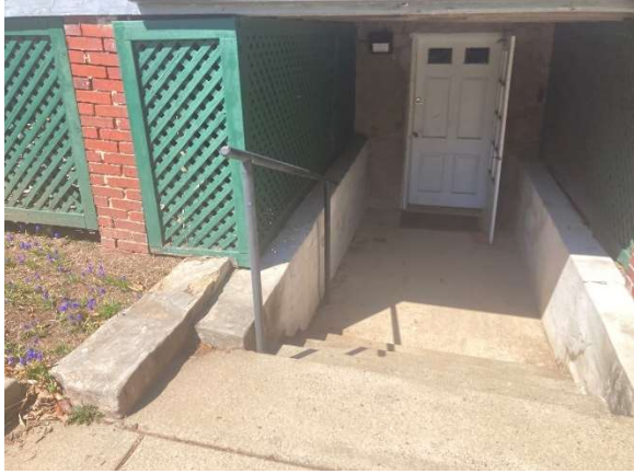
Areaway to basement, showing existing (noncurrent-standard) pipe railing
