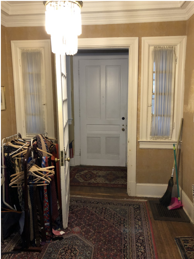
Existing Front Door interior. Existing interior vestibule door and windows to remain.
