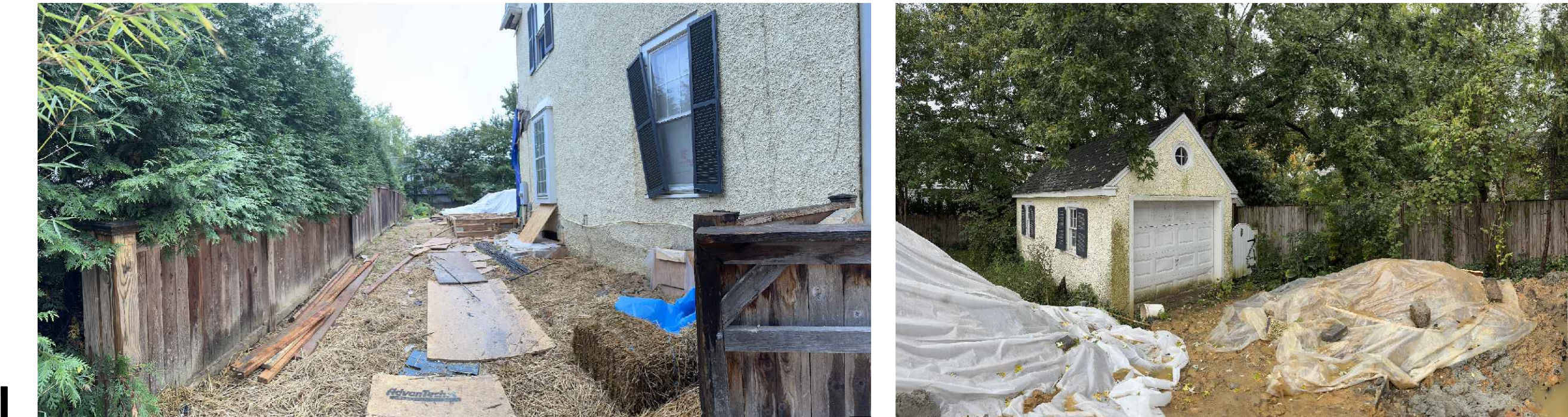
VIEW FROM FRONT LEFT CORNER OF HOUSE TOWARDS BACKYARD | VIEW FROM BACK OF HOUSE TOWARD EXISTING GARAGE
