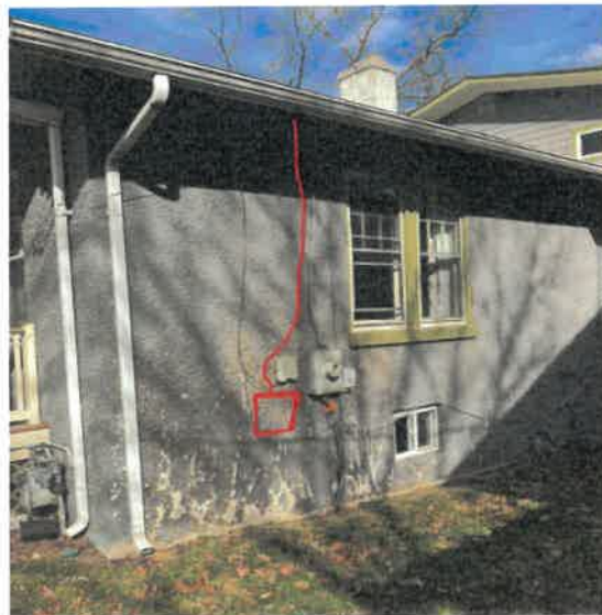
Seavey Utility Side Example After Installation
