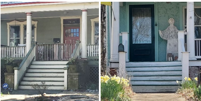
Figure 3: View of the similar stair configurations at 7219 Maple Avenue (left) and 7109 Carroll Avenue (right), 2023.
