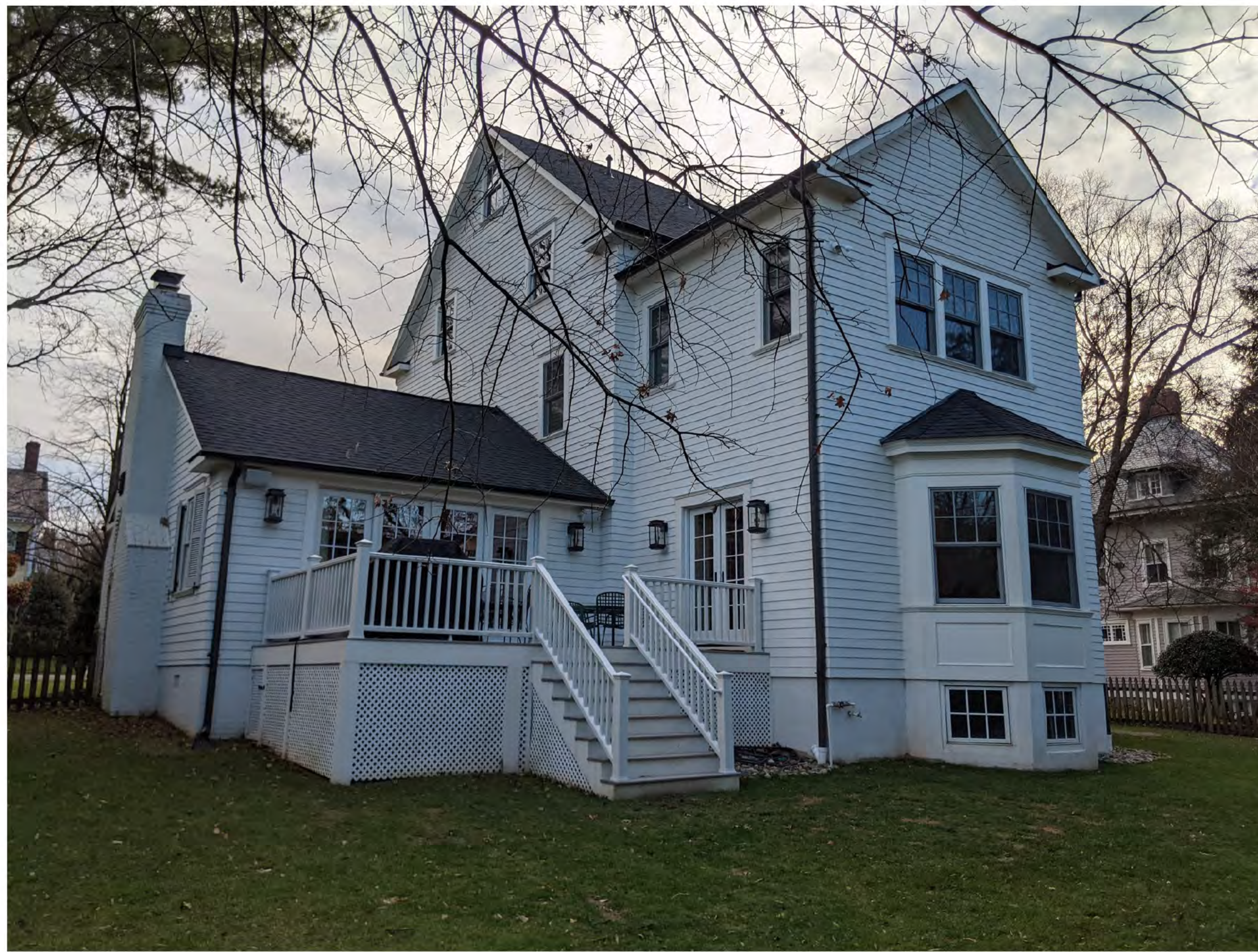
1 11 E. LENOX STREET AREA OF WORK, NORTH ELEVATION A702 NOT TO SCALE
