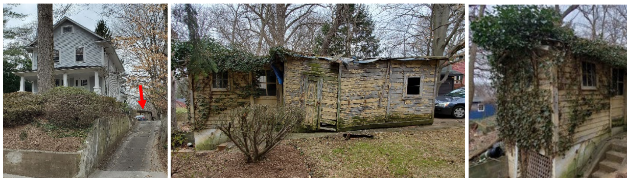
Figure 2: View of the accessory structure from Maple Avenue (left), the south elevation of the accessory structure (center), and the west and south elevations of the accessory structure (right). The red arrow points to the location of the subject structure.
