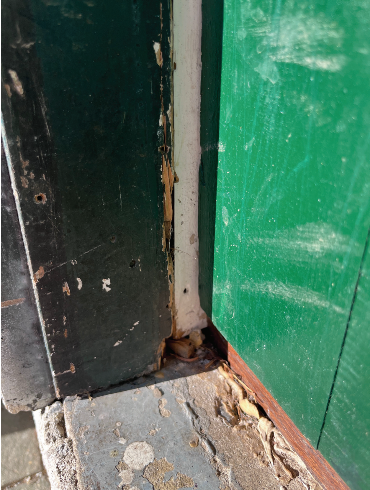
Close up of damage to wood and cement threshold of exterior door to entryway
