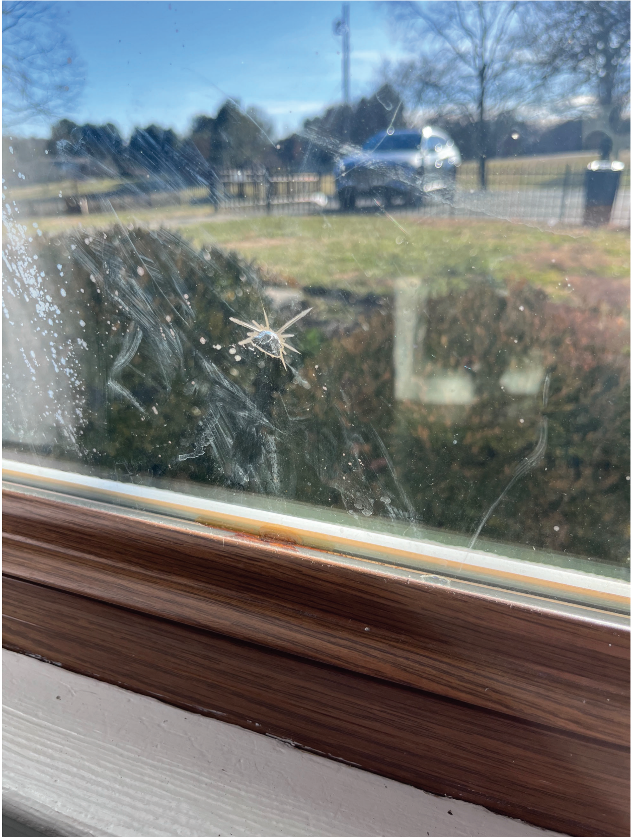
Damage to glass on second window in living room
