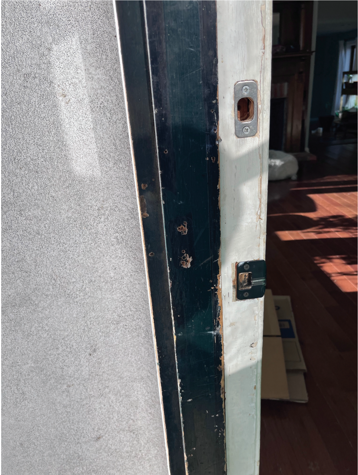
Weathering of wooden frame for exterior door to entryway
