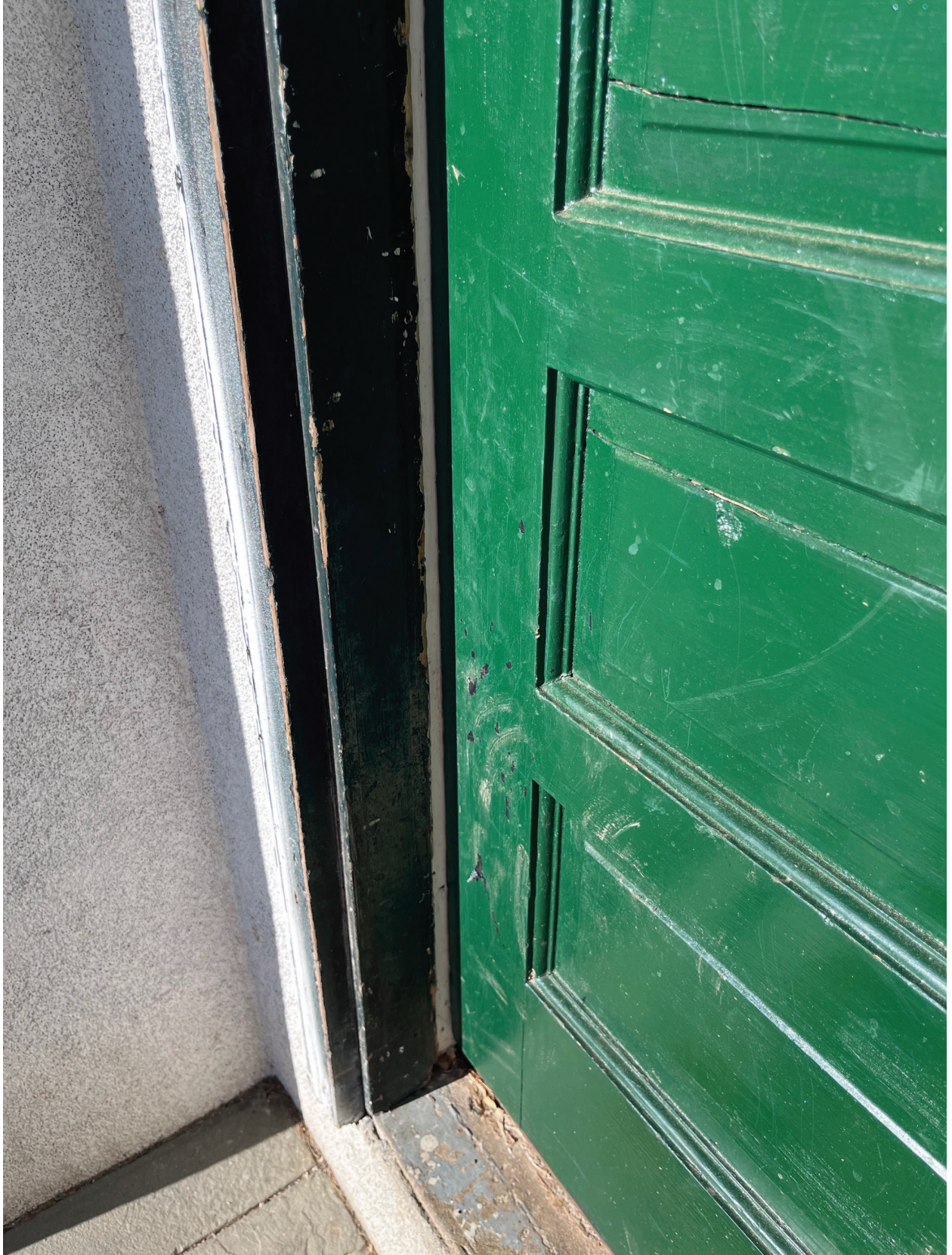
Weathering on wooden frame and door does not lie flush with frame. Cement threshold cracked.
