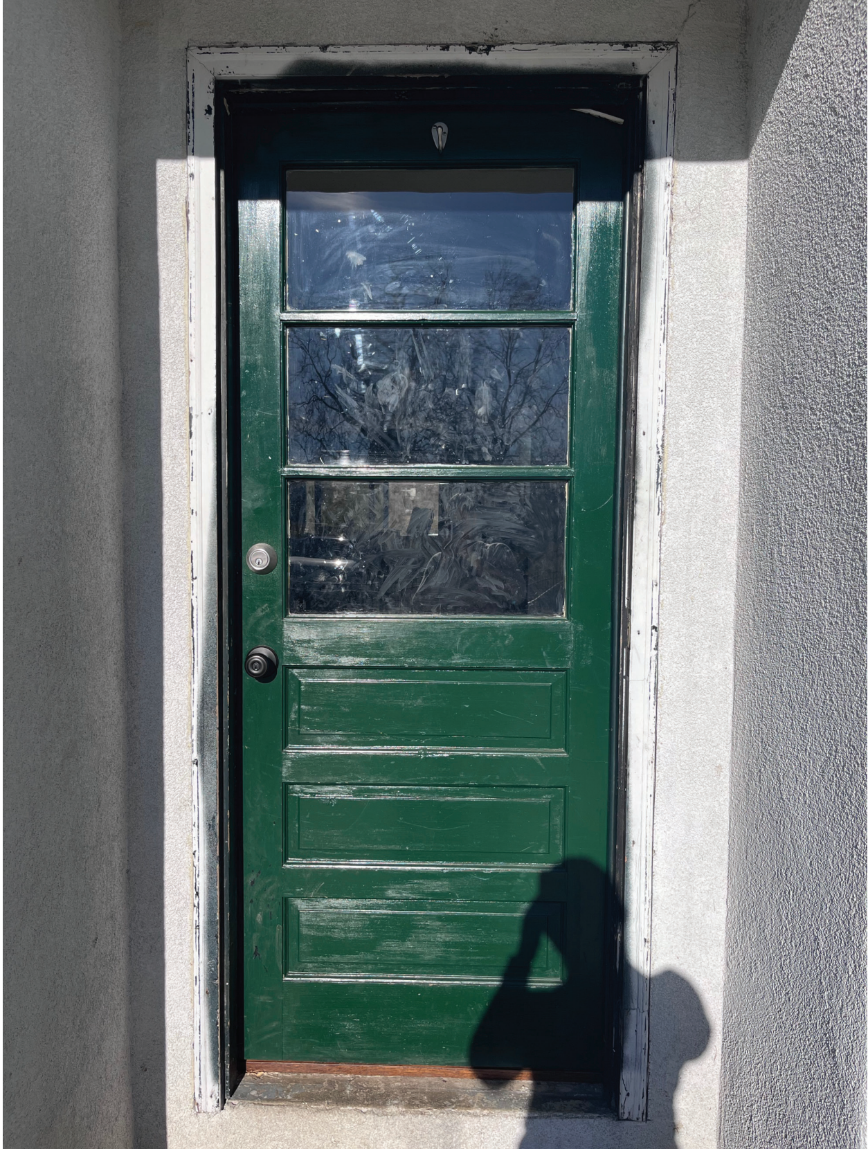
Exterior front door with wooden frame painted white (storm door had been damaged in windstorm and removed).
