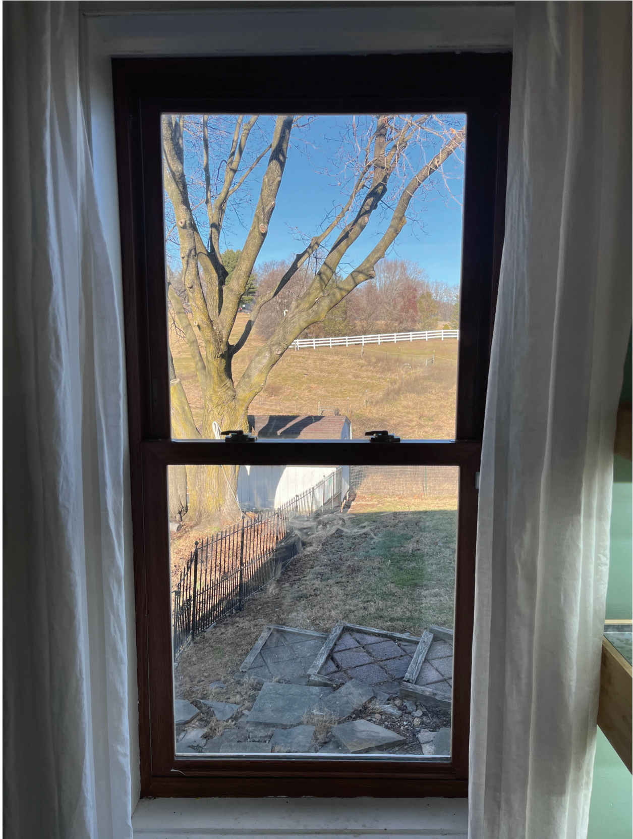
View of window with damaged vinyl frame
