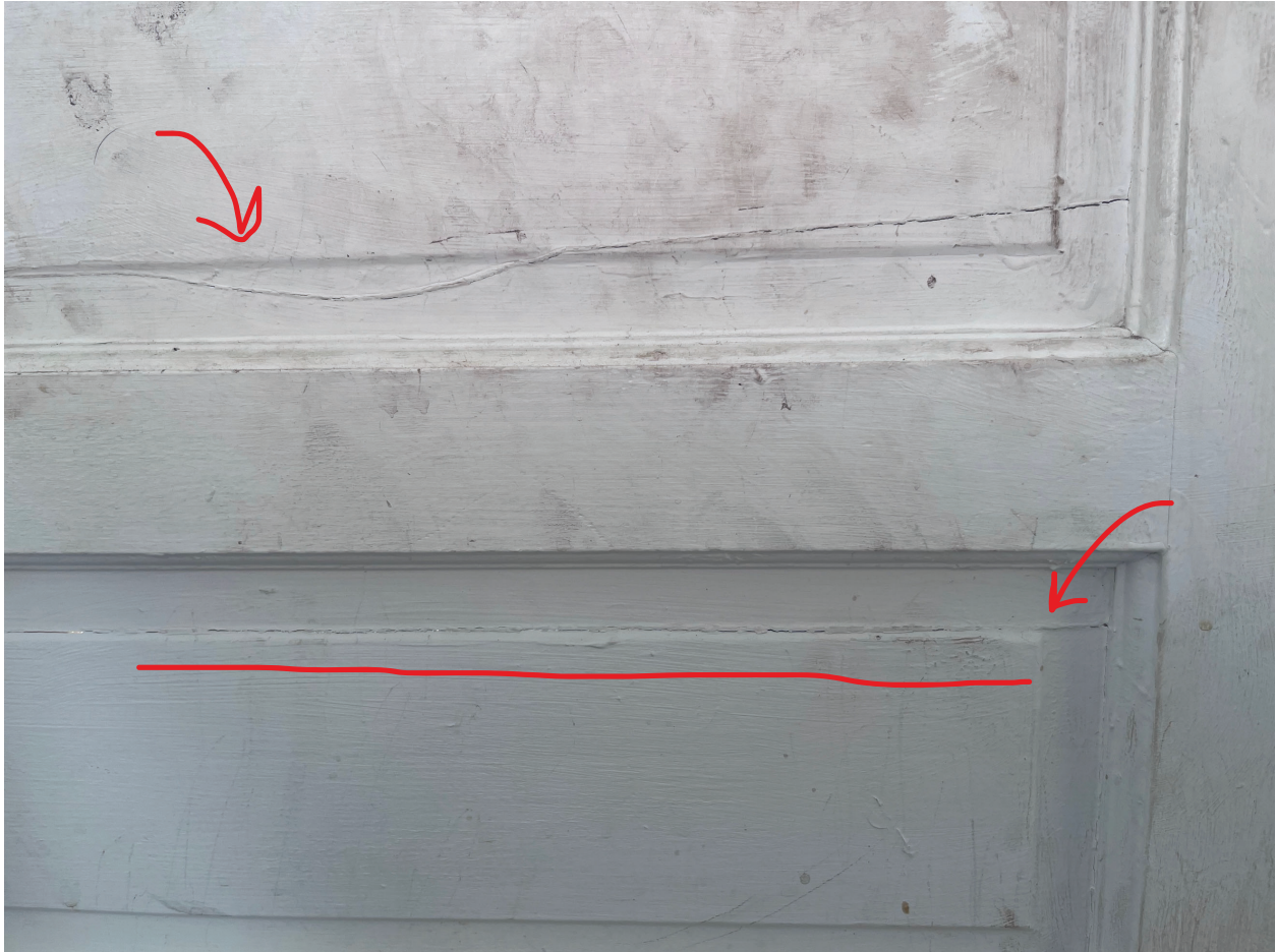
View of cracks covered by painter's tape in photo above. Second crack is underlined in red
