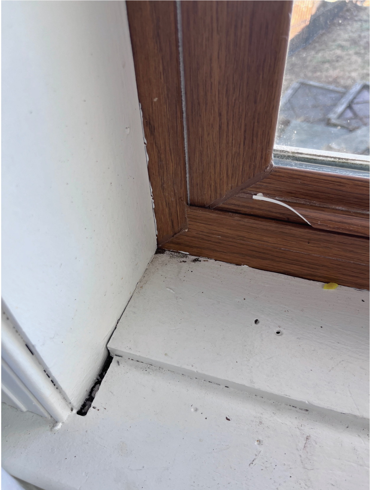
Damage to window vinyl frame and warping around window sill
