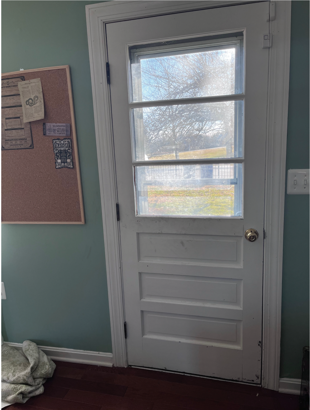
Second exterior door missing a pane of glass on lower third (replaced with plexiglass sheet). Door does not fit properly within frame and lets in significant amount of air through the bottom.
