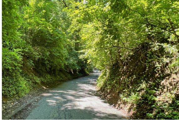
Views looking south of high banks on both sides of Swains Lock Road
