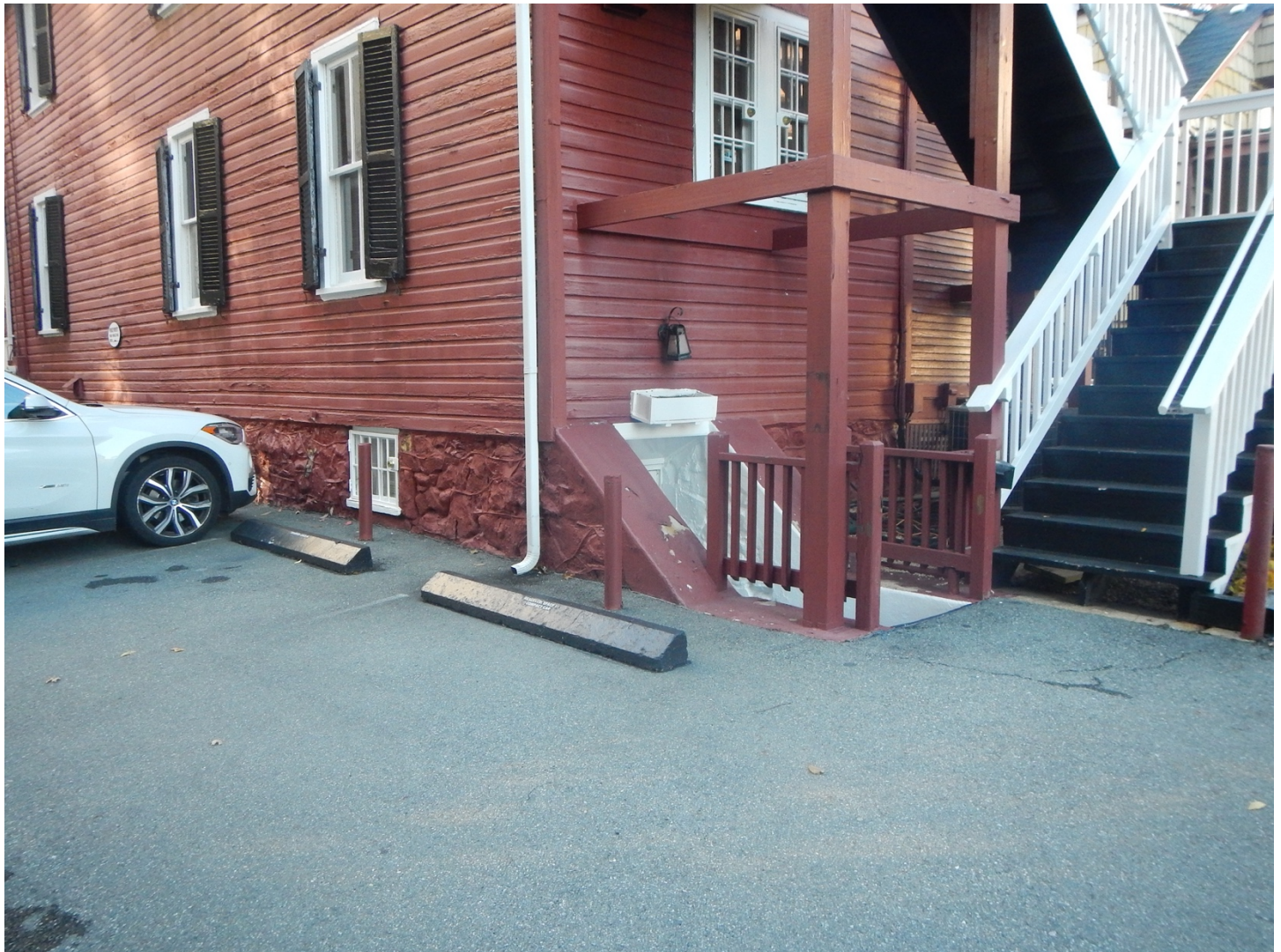
Figure 11. Detail of Basement Entrance and Foundation Materials at rear of Joseph F. Pyles House, Facing Northeast (November 15, 2021).
