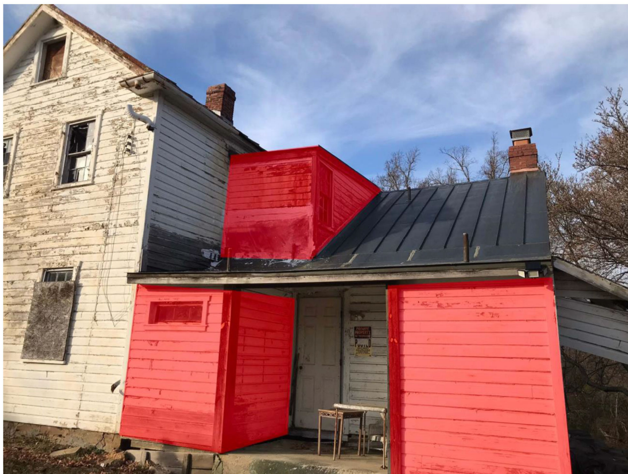
Fig. 3: Rear of the eastern section of the historic house, with previous alterations/bathroom additions tinted red.
