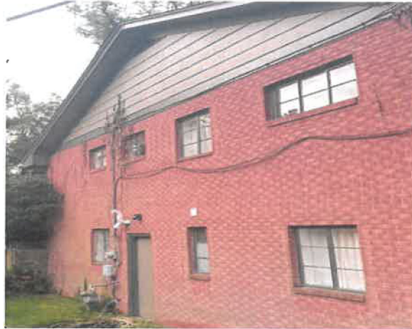
Utility Side Before Installation
