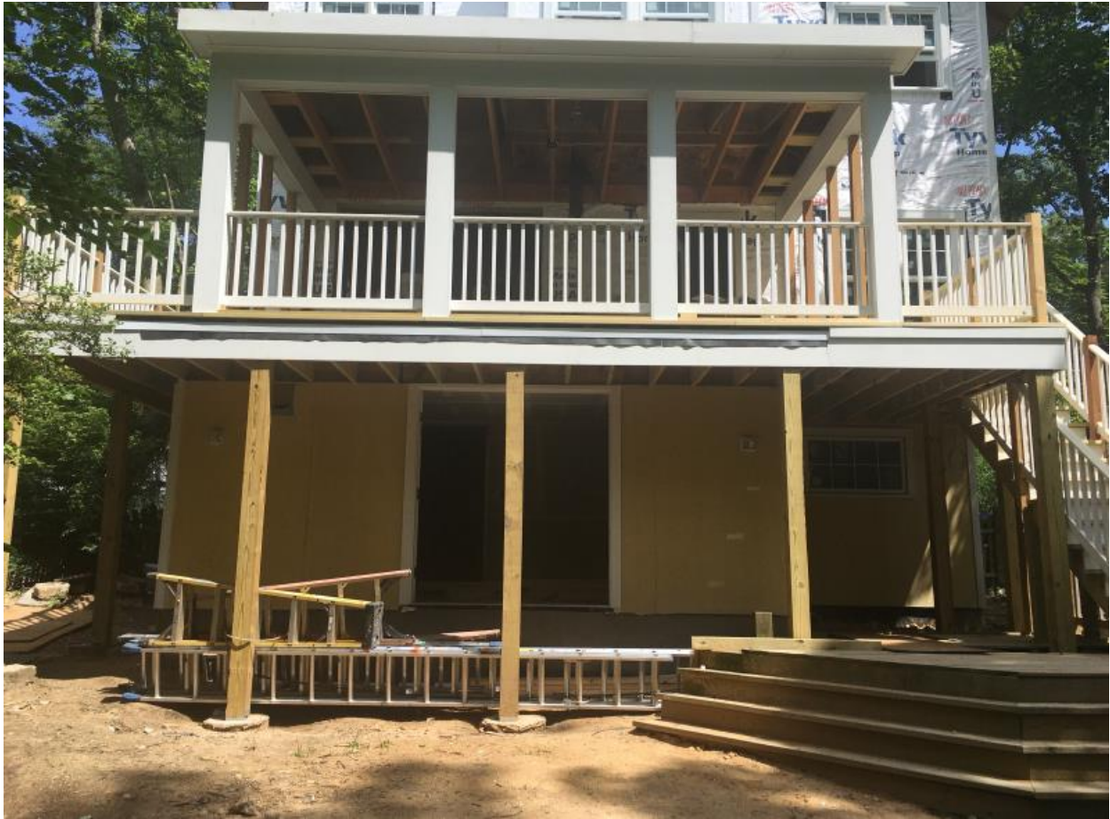
Figure 2: Rear of 7306 Maple Ave. under construction showing the drop in grade from the rear door.
