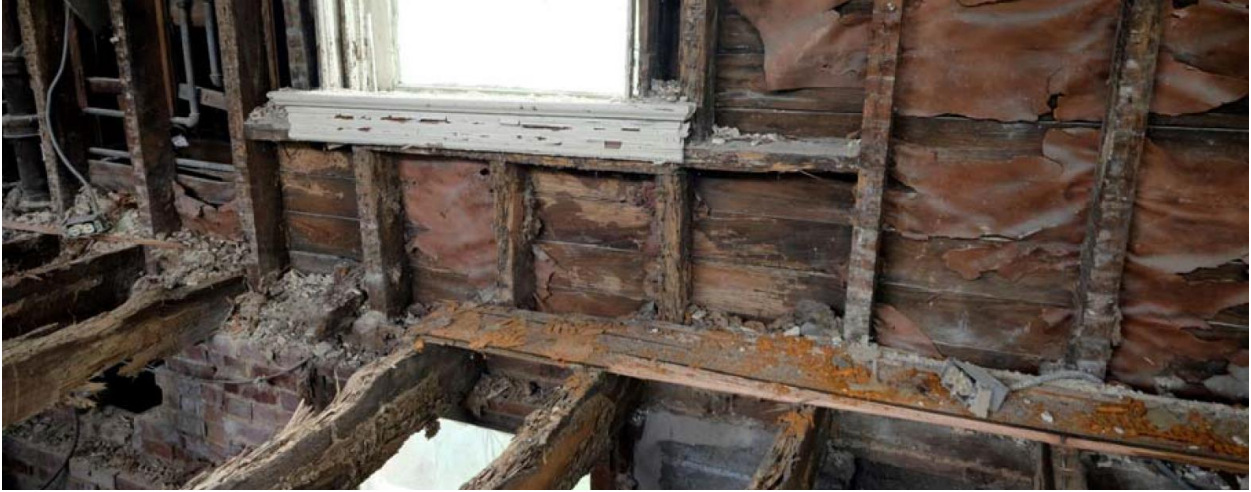
Figure 2: Detail of the termite damage done to the house framing and window frames.
