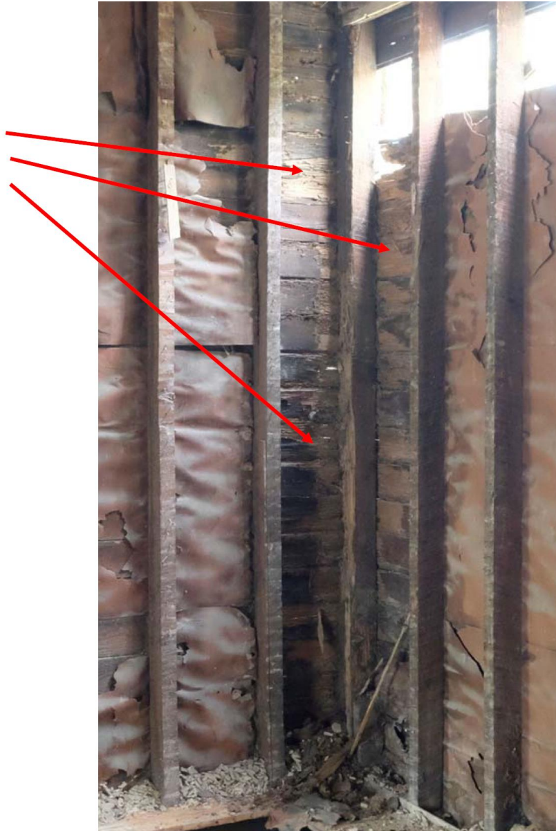
Figure 3: Termite damage at the exterior corner of the house showing the termite damage.
