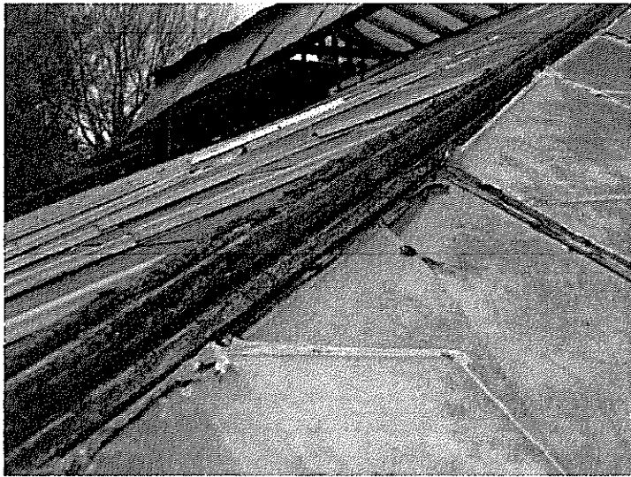
Photo 6 Rotting hip beam
