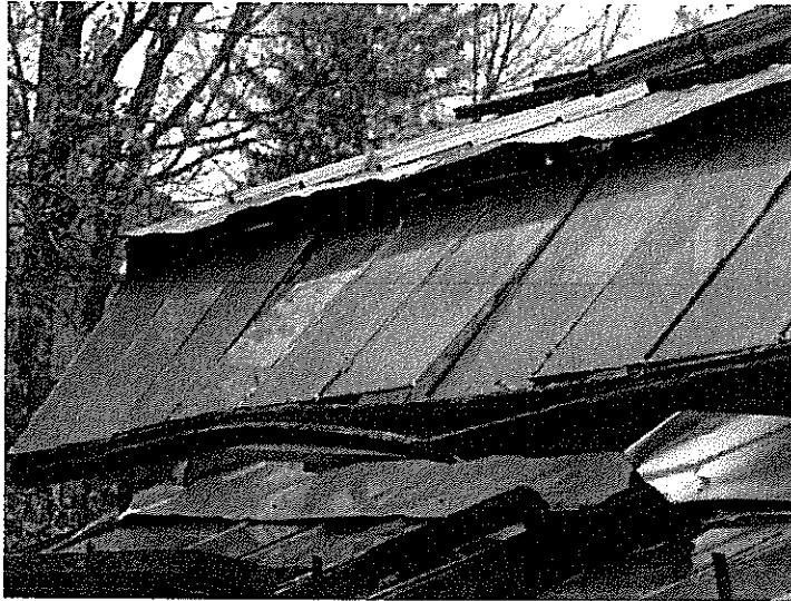
Photo 7 Loose glass panes and rotten lumber in awning window
