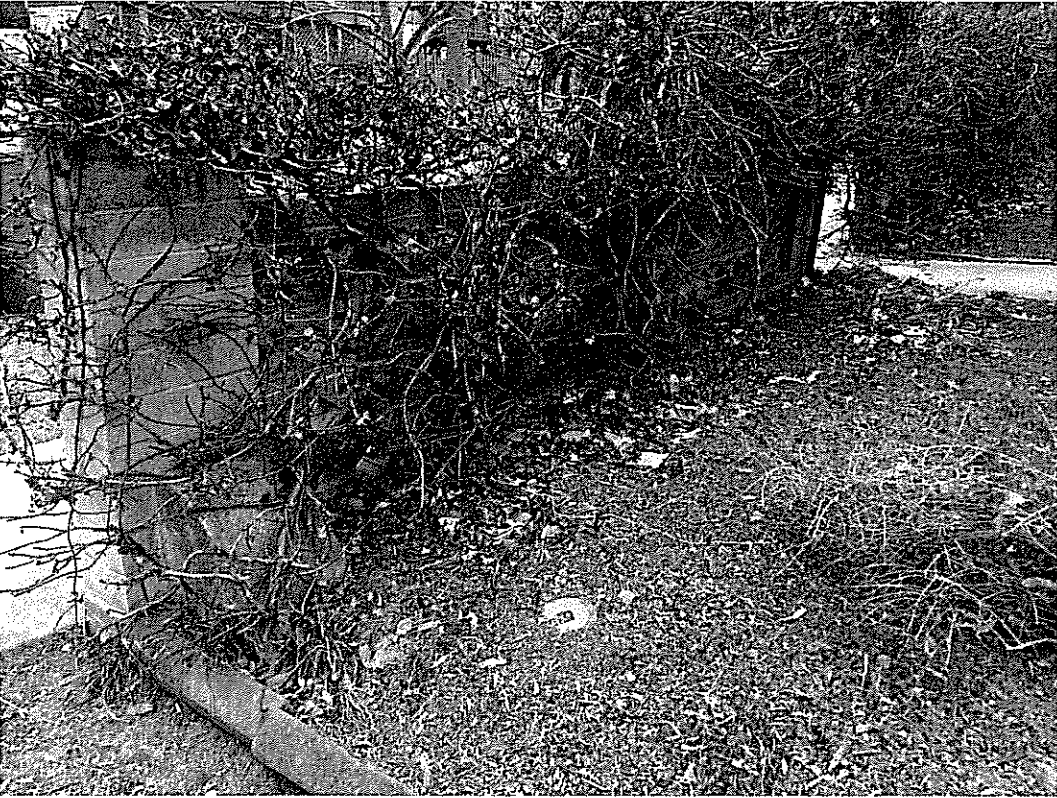
Detail: Back of CMU wall, taken from yard towards street
