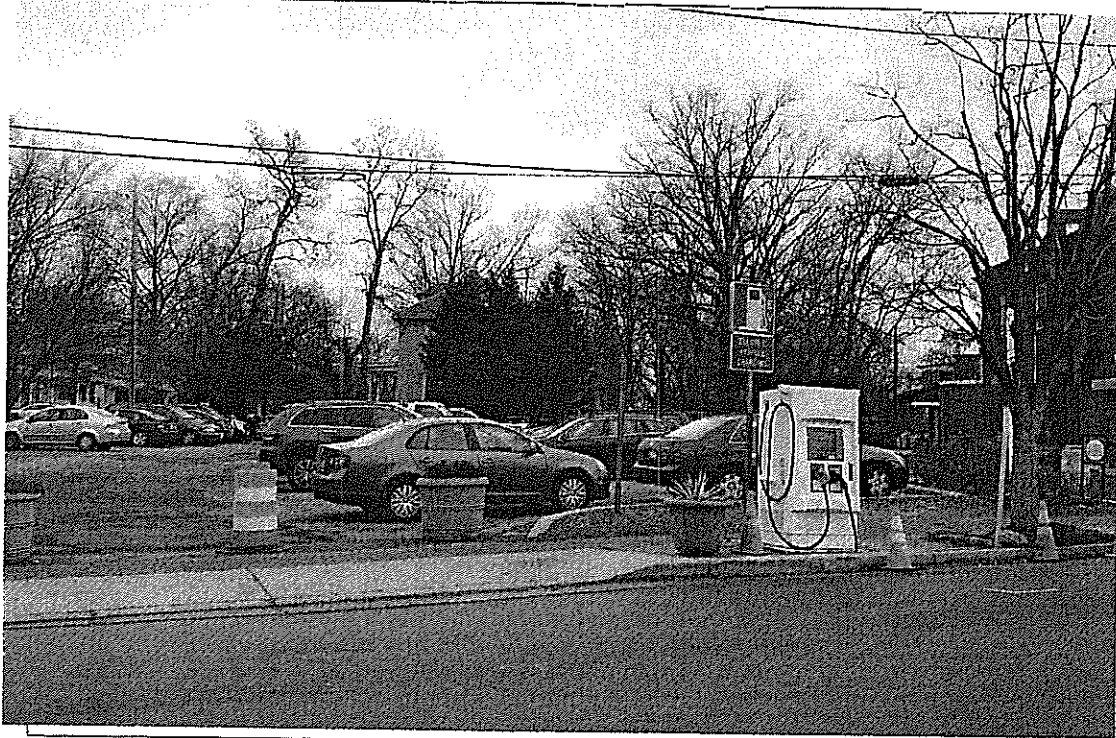
Detail: View of the southbound public right of way and parking spot on Carroll Ave. Station color can be changed to blend in with surroundings or left clean as is.
