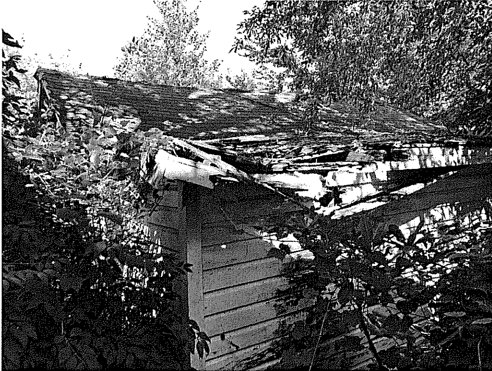
Figure 1: Roof failure at the rear of the garage
