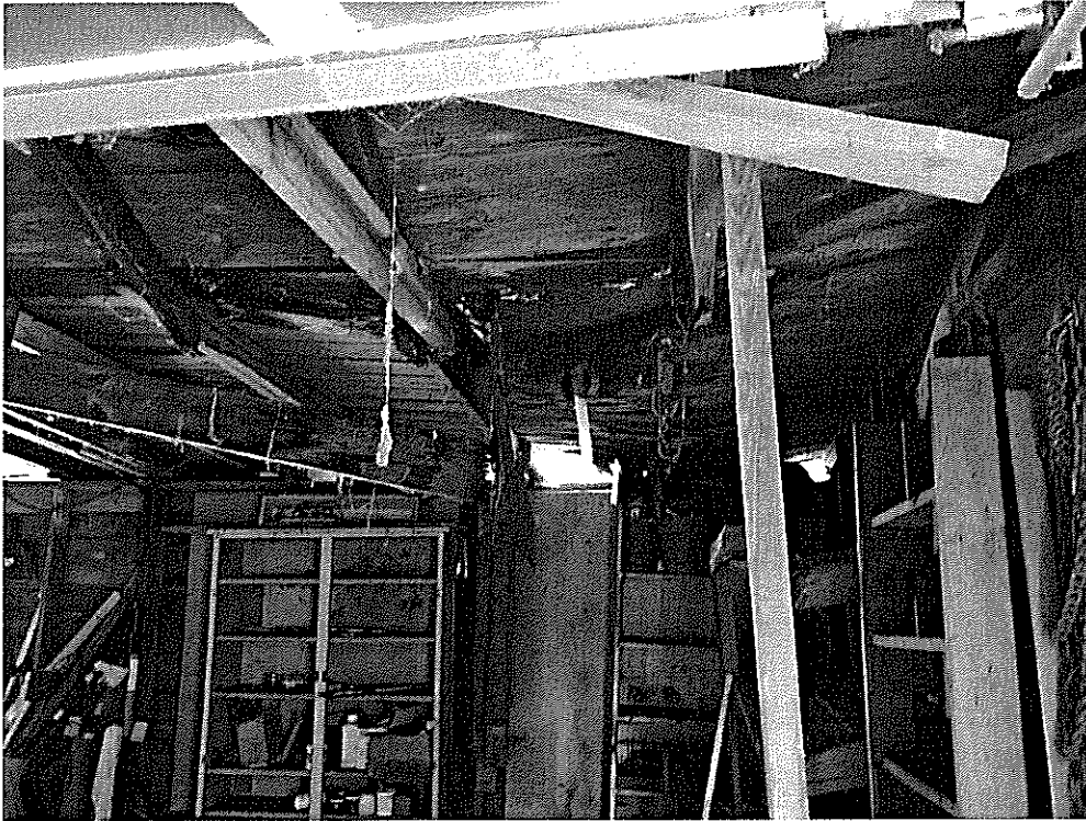
Figure 2: Interior rafter failure
