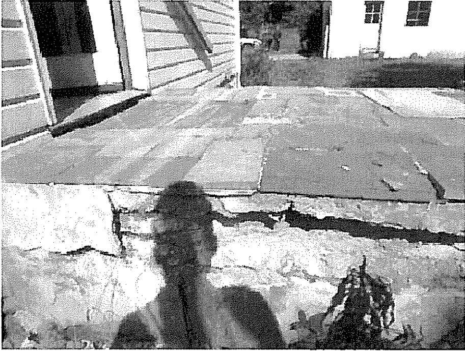
Photo 4: detail of east side of stoop showing wood trap door immediately in front of open door.
