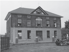
The HPC issued a Stop Work Order after being notified that the exterior had been altered without a Historic Area Work Permit.
