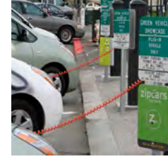
Electric Vehicle Charging Stations
