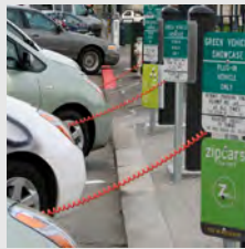
Electric Vehicle Charging Stations
